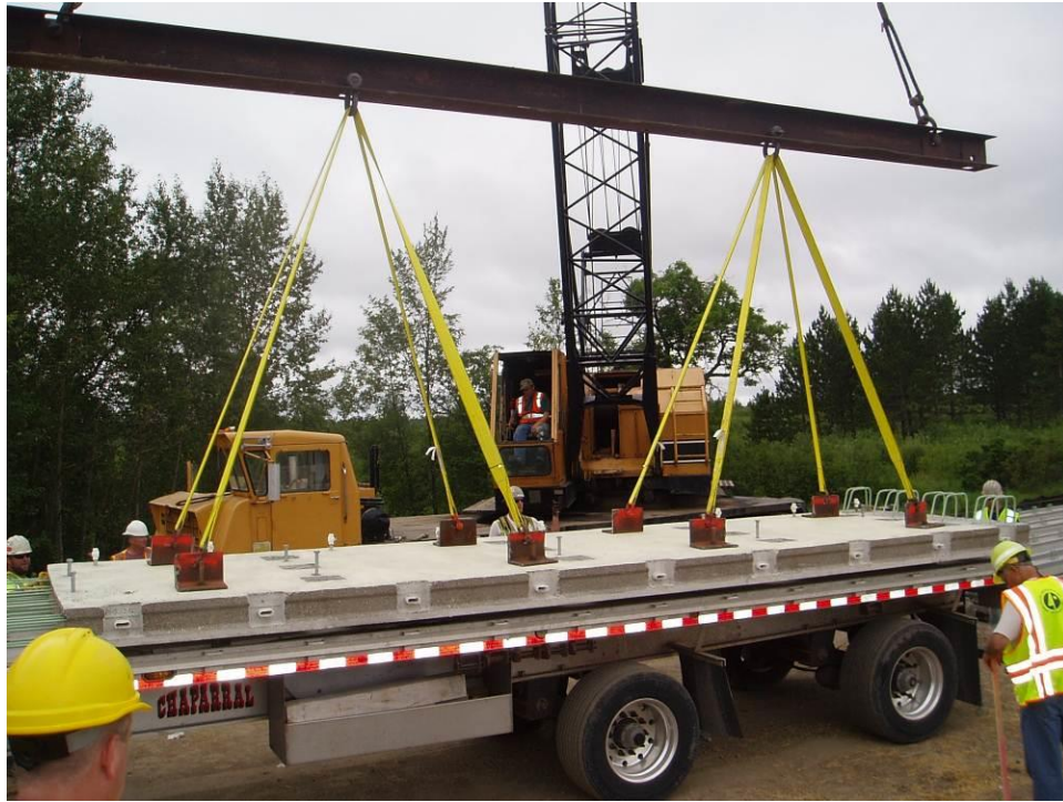
Figure 22. Lifting the deck panels from the flatbed truck using crane and lifting hardware.
