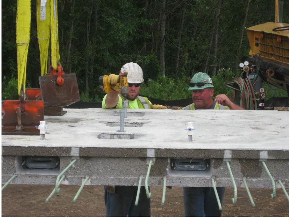
Figure 24. Passing the leveling bolt through the cast sleeve and screwing through the cast nut.
