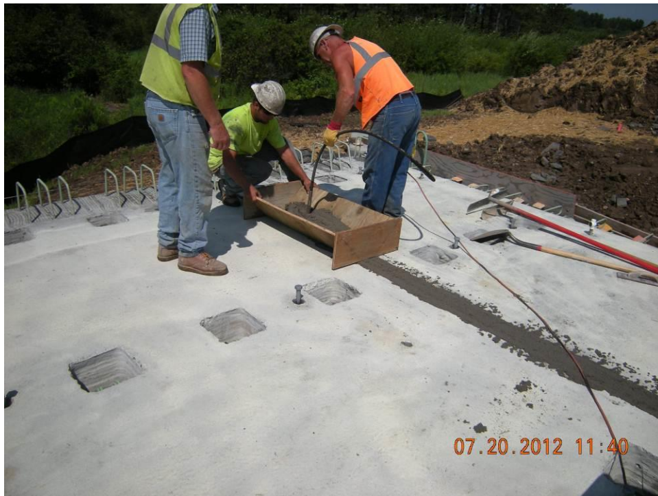
Figure 51. Vibrating the grout into the transverse keyway joints and post-tensioning duct splice blockouts.
