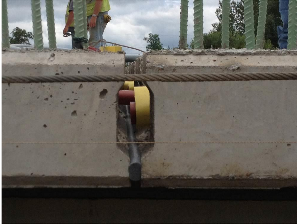
Figure 40. Side view of backer rod in place. The panels were placed such that they were in tight contact with the backer rod separating them.
