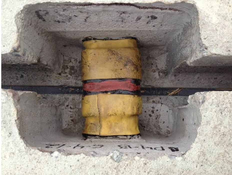
Figure 44. Heat shrink sleeve tightly covering each connection of the corrugated plastic ducts. It prevents post-tensioning grout from escaping at the connections.
