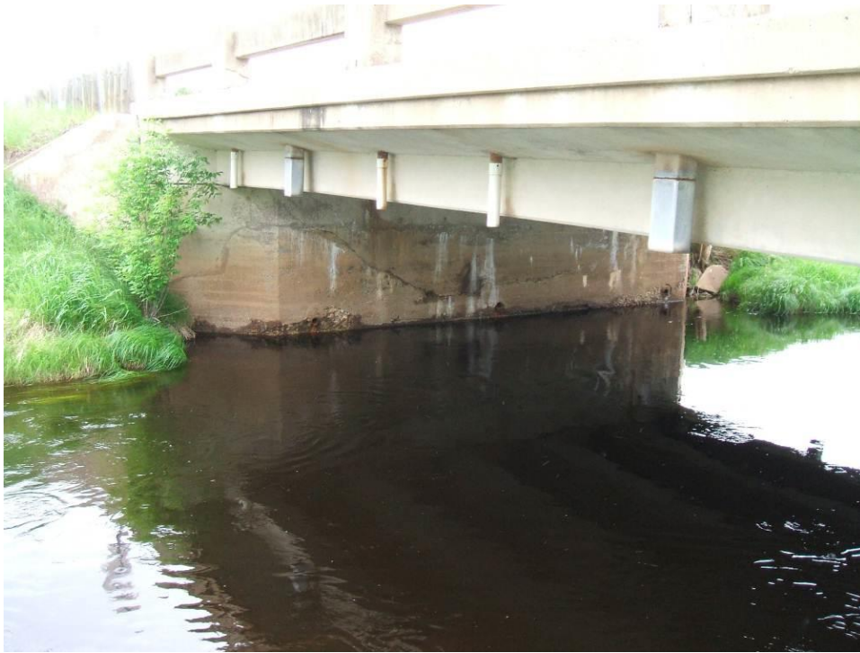
Figure 4. Deterioration of bridge 6603 north abutment wall.
