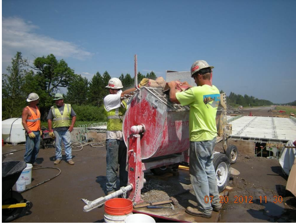
Figure 48. Mixing the grout for the keyway joints and post-tensioning duct splice blockouts.
