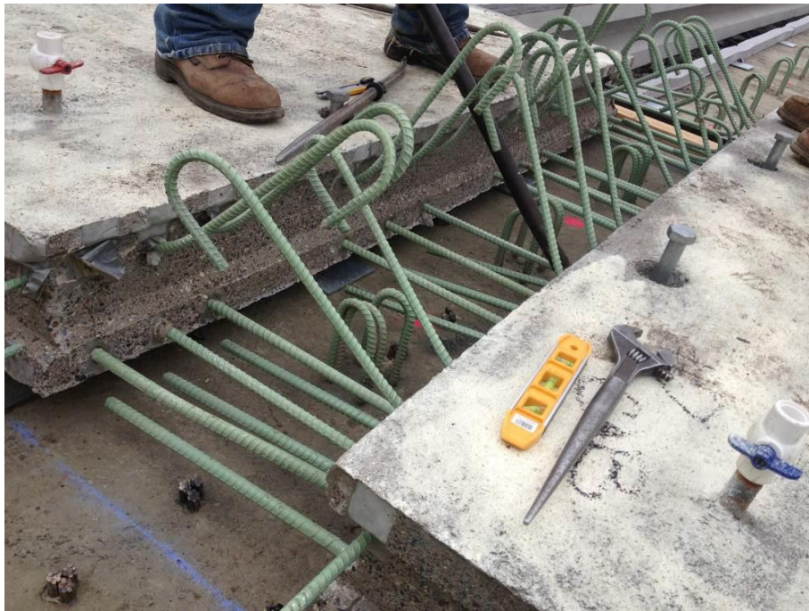
Figure 45. Reinforcing steel protruding at the 18-inch longitudinal joint.
