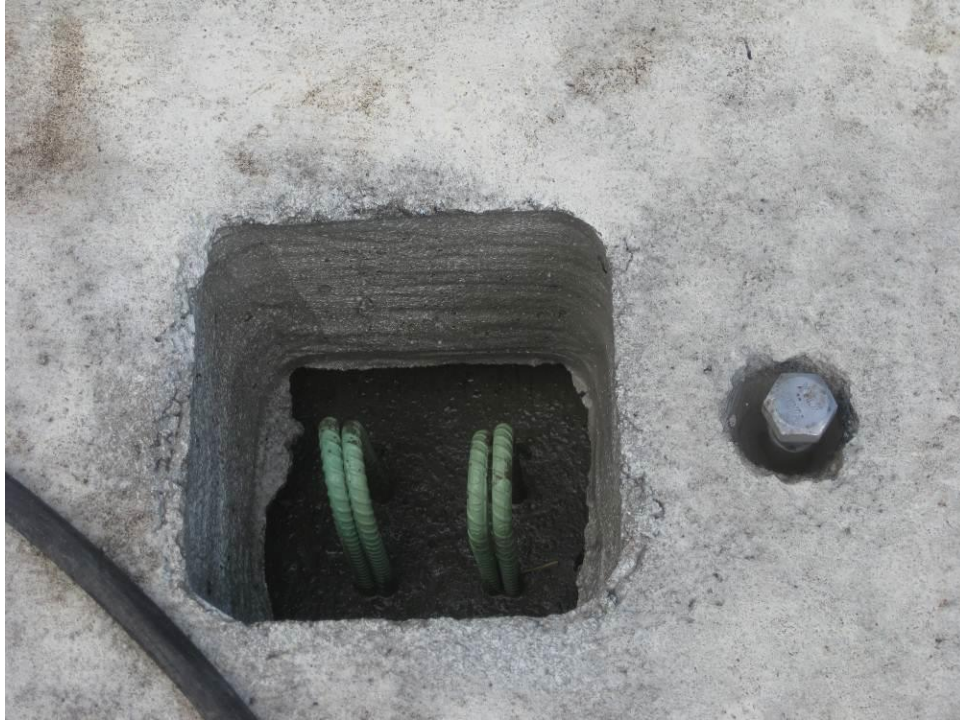
Figure 28. Shear breakout to be filled with grout to provide composite action between the girder and the deck (to the right is a leveling bolt).
