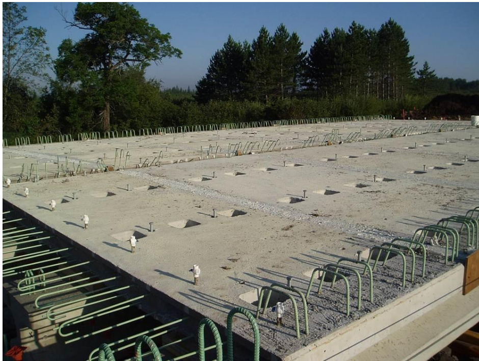
Figure 57. Bridge 69071 after placement of grout in the transverse deck panel keyway joints and post-tensioning duct splice blockouts.
