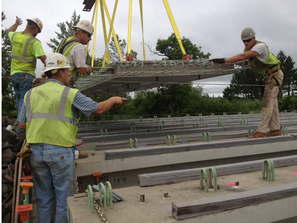
Figure 26. Placement of the deck panel onto the concrete girder (horizontal cable shown is the safety harness for crew on top of the girder).
