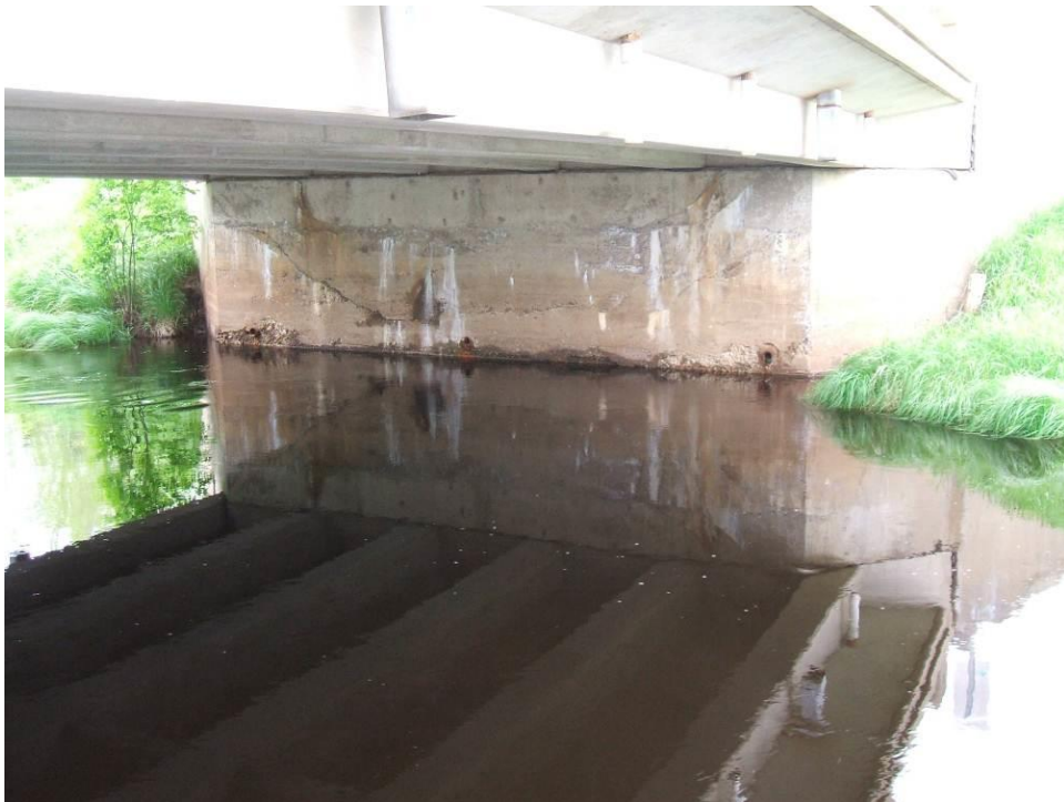
Figure 3. Deterioration of bridge 6603 south abutment wall.
