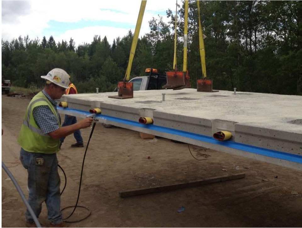
Figure 38. Spraying the bottom of the panel joint with adhesive to install the backer rod.
