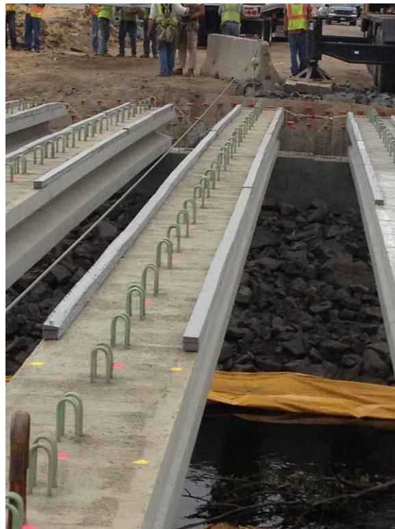
Figure 16. Placement of the haunch-forming material at the edges of the concrete girders.
