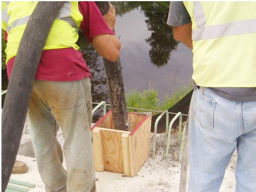
Figure 69. Close-up of grouting the haunches and the shear pocket blockouts by pumping extended grout through the shear pocket blockouts.
