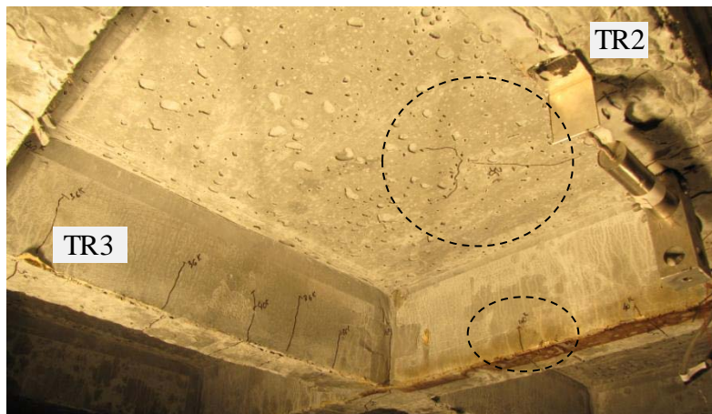
a) Cracking on the bottom surface of the slab and on a longitudinal rib
