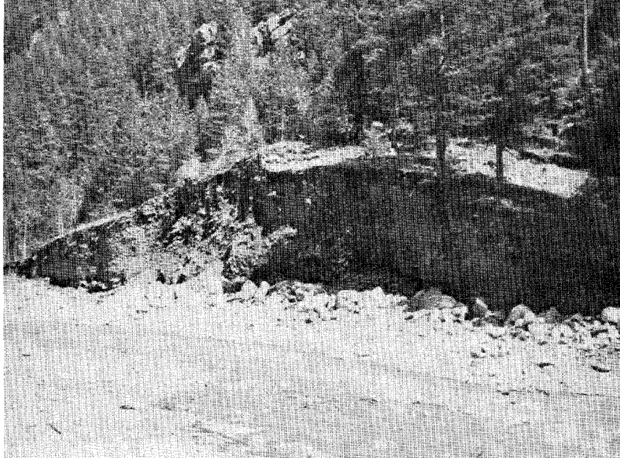
Figure 23. Severe Toe Erosion Along Debris Fan.
