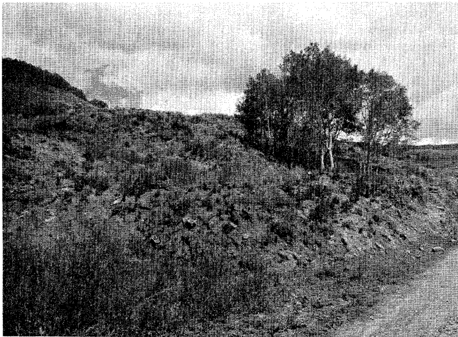
Figure 27. Trees Growing in Isolated Area Due to Drainage Patterns Contributing to Slope Failure.
