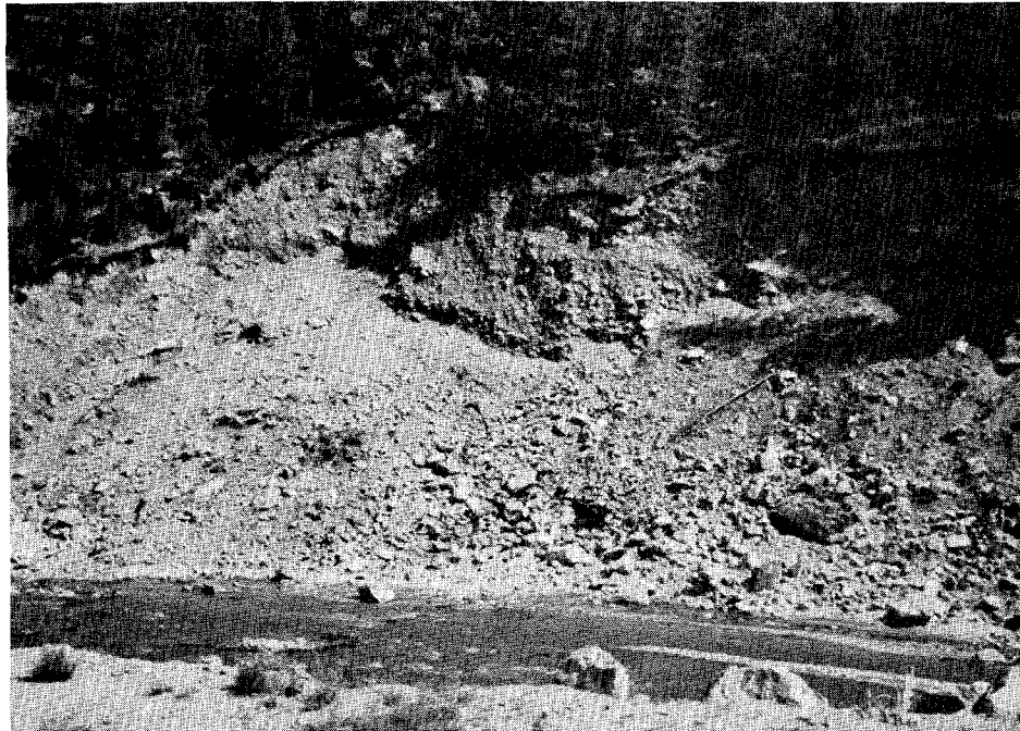
b. Slope Failure Near Glen Comfort.
