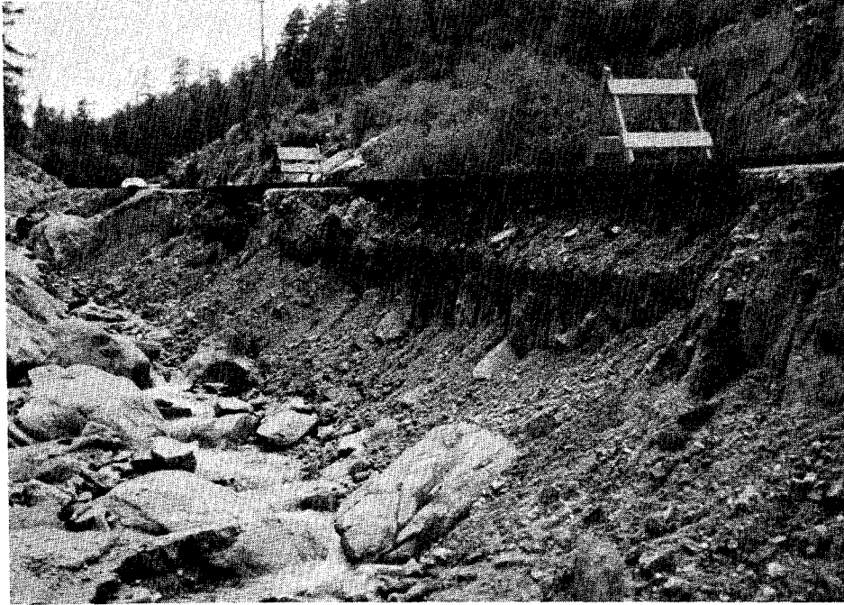
a. Undercutting of Pavement Along North Fork Big Thompson River.
