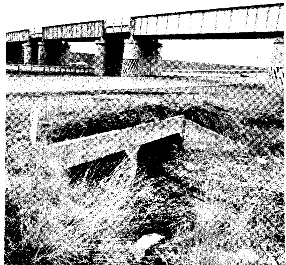
Figure VI-15--Sediment deposition in culvert.
