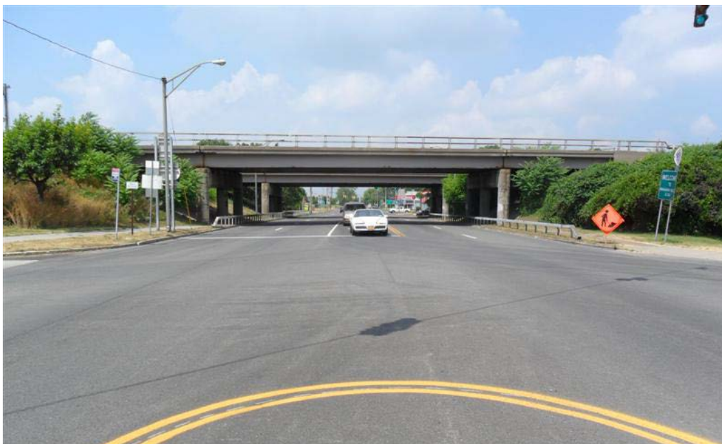
Figure 4. Photo. Elevation view of bridges with substandard underclearance.
