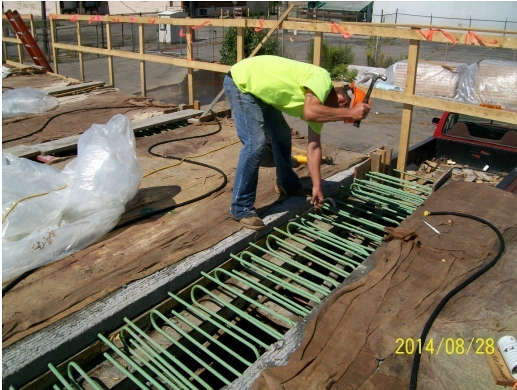
Figure 22. Photo. Correcting rebar conflicts between adjacent modular units.
