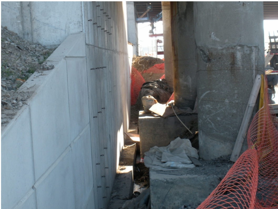
Figure 17. Photo. Tight space between existing and new units.
