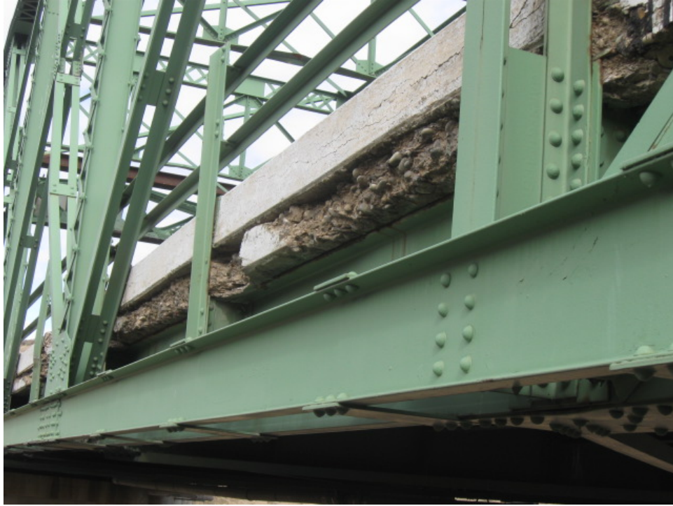
Figure 3. Deterioration of bridge 0700 deck.
