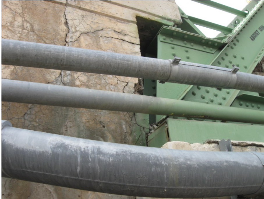
Figure 5. Deterioration of bridge 0700 abutment wall.
