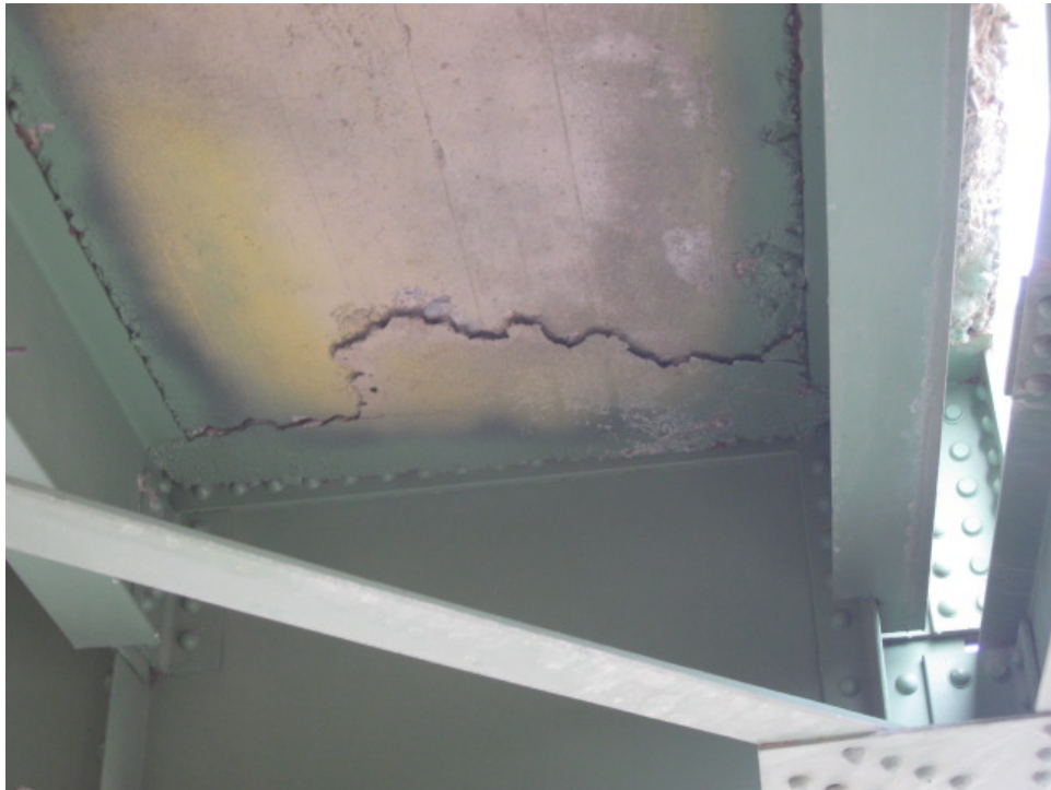
Figure 4. Deterioration of bridge 0700 deck.
