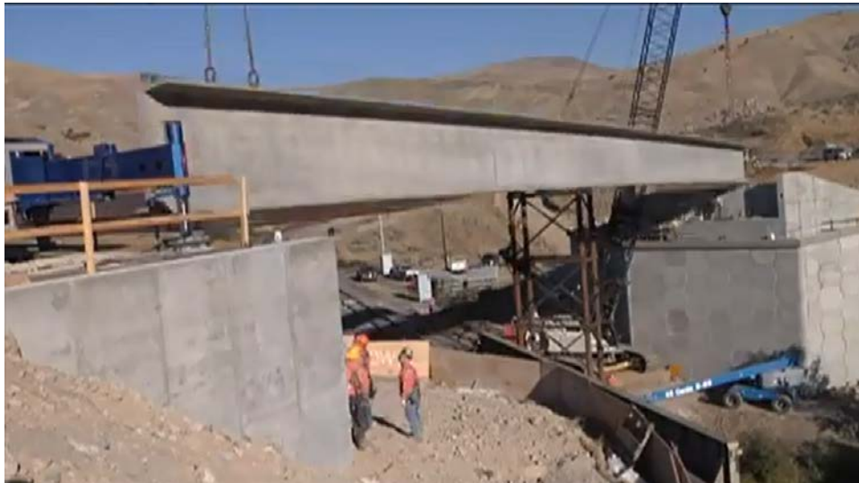
Figure 32. Girder transferred from the temporary support to the bent abutments during construction of the superstructure.
