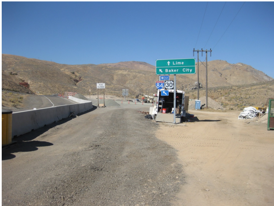
Figure 60. Closure and barriers detouring traffic on to WB I-84 at the south end of the project.
