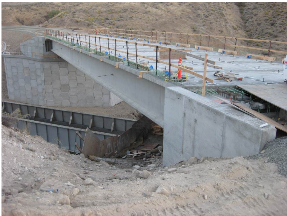
Figure 38. Long view of the girder and deck from south end of the bridge following installation of all prefabricated bridge deck panels.
