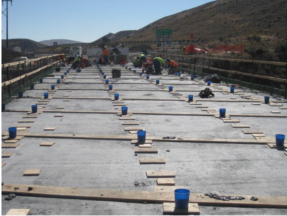
Figure 55. Long-shot view of bridge deck showing top-formed filled areas of UHPC to prevent overflowing. The placement concludes at the chimney to allow for slight overpressure on the field-cast UHPC which assists in ensuring that the connection space is fully filled.
