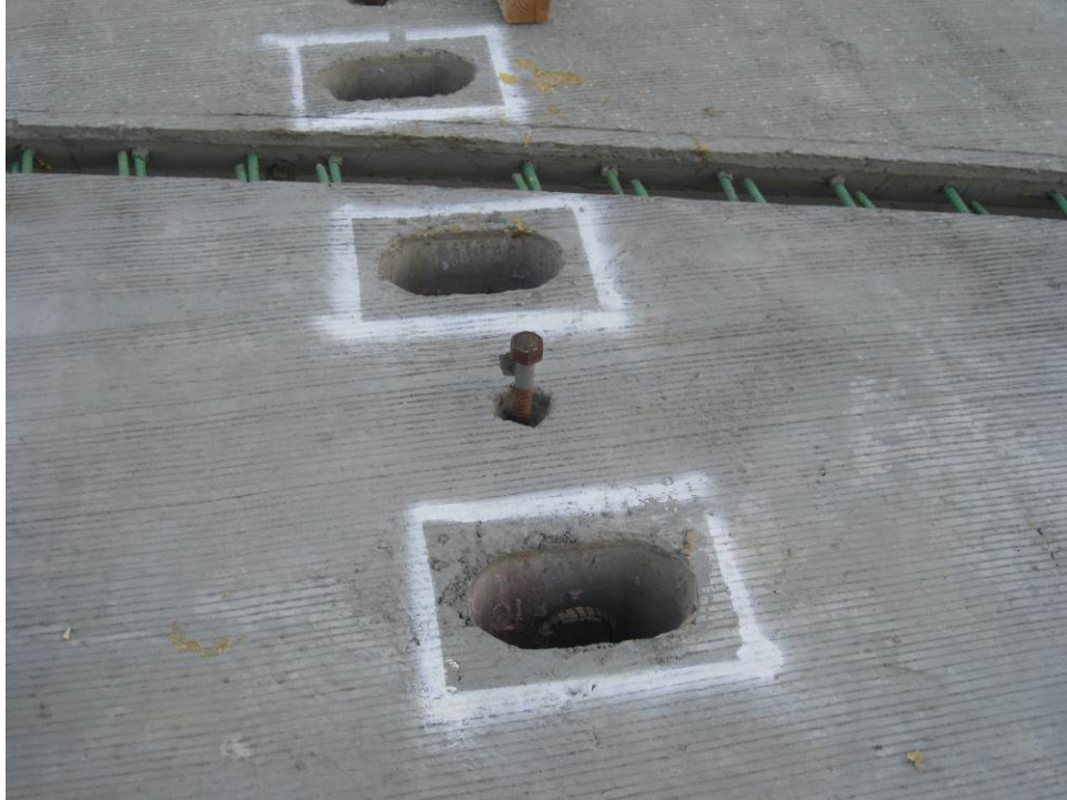
Figure 43. Medium view of the deck panel shear pockets placed over reinforcement from the girder. Also in the view is a leveling bolt and the joint between the deck panels.
