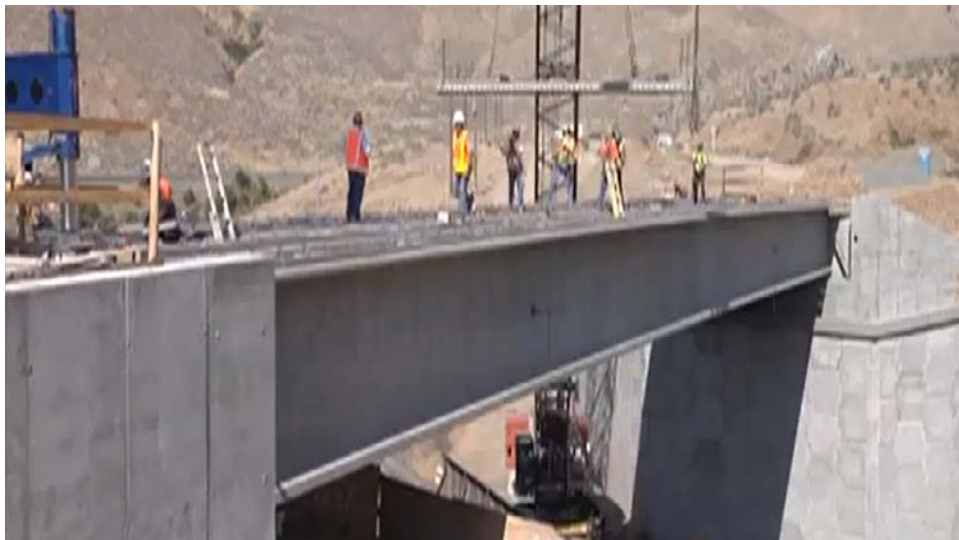
Figure 34. Installation of the prefabricated bridge deck panel (P8) during construction of the superstructure.
