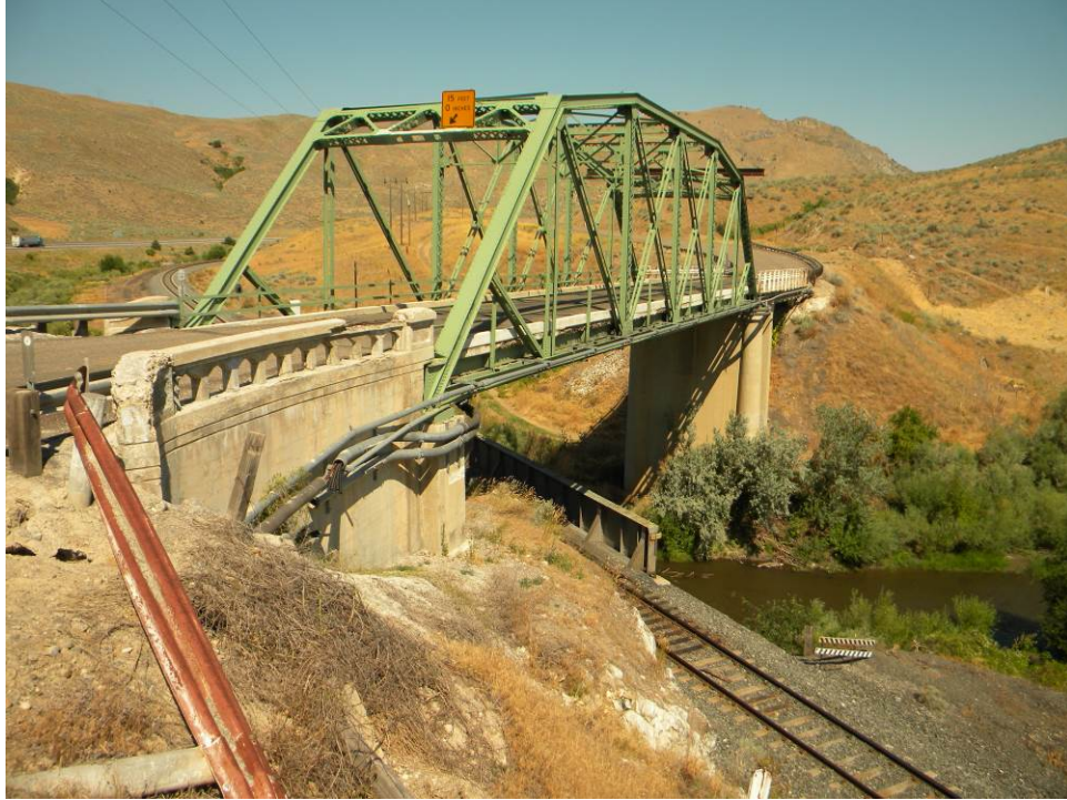
Figure 1. Overview of condition of existing bridge (#0700) over Burnt River and an active railroad track.
