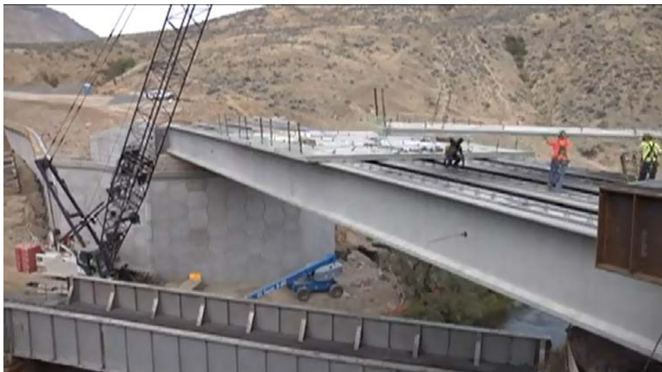
Figure 36. Continuing installation of the prefabricated bridge deck panels during construction of the superstructure.
