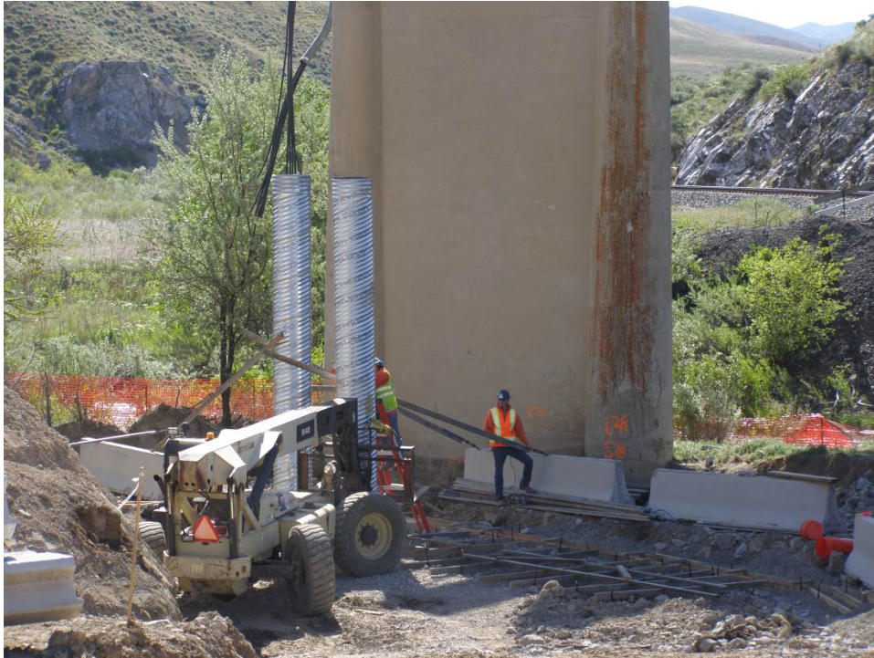
Figure 23. Installation of corrugated metal pile spacers for building the substructure and MSE retaining wall.
