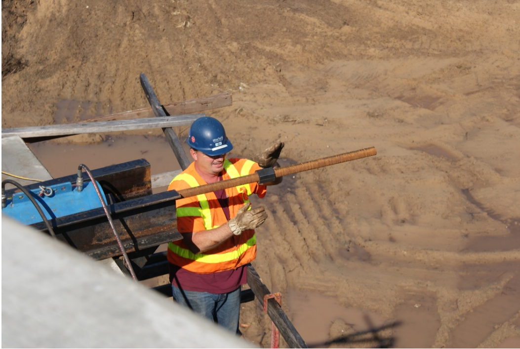
Figure 17. Photo. Threaded nut used to lock rod to ram prior to pull.
