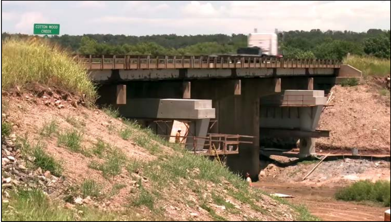
Figure 5. Photo. New piers and caps in place below and between existing piers.
