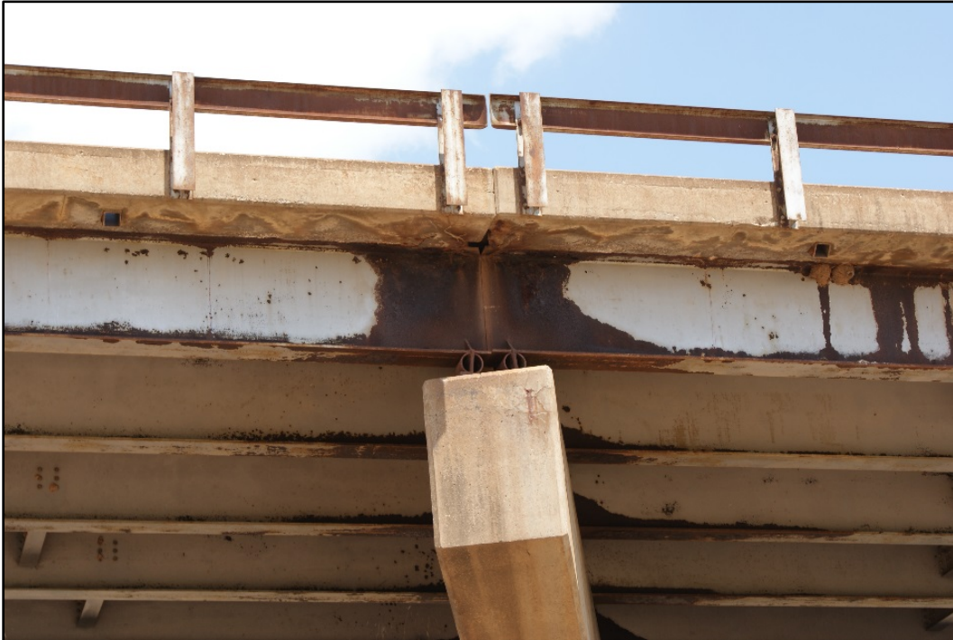
Figure 3. Photo. Deteriorated steel and support mechanisms on existing bridge.
