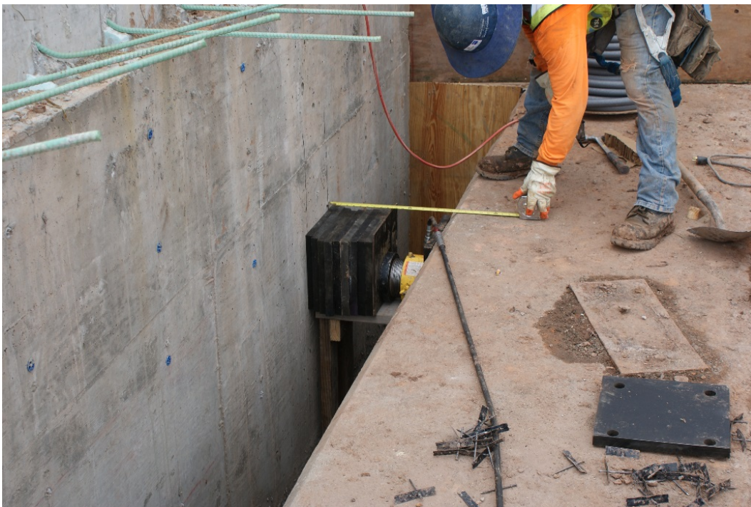
Figure 18. Photo. Air-operated jack placed between abutment and deck slab to provide adjustment between sections.
