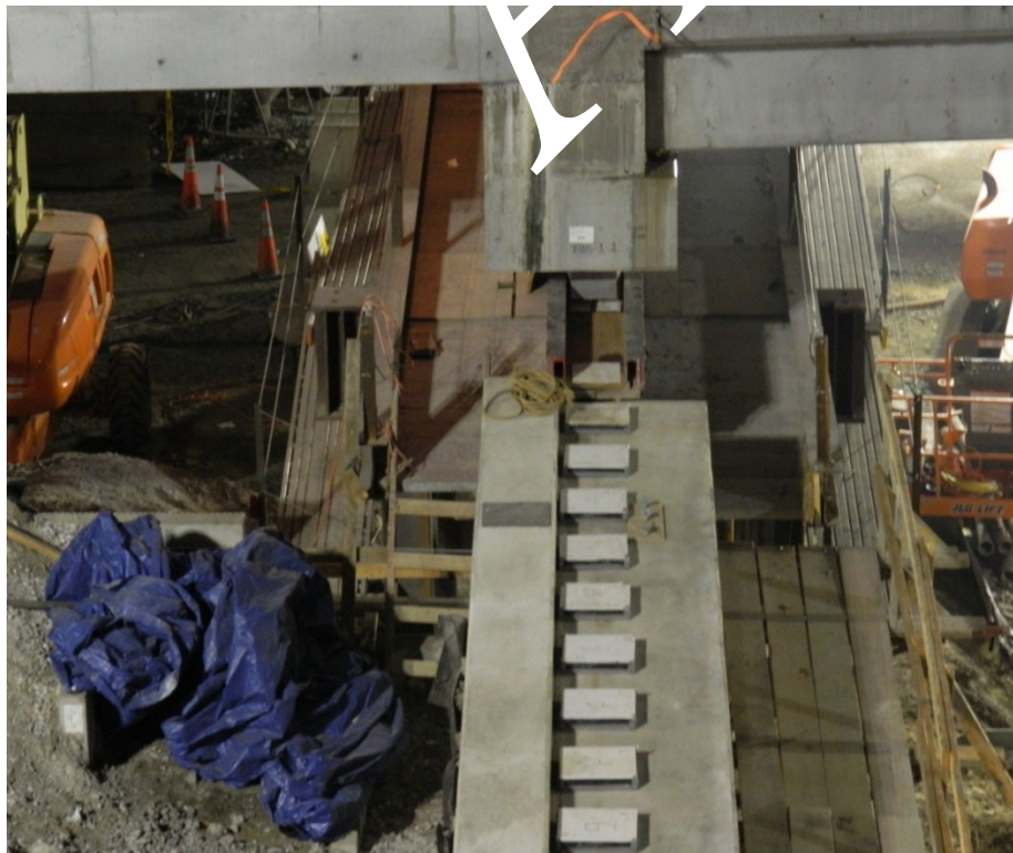
Figure 38. Photo. PTFE pads on sleeper slab to facilitate sliding at end of approach slab.
