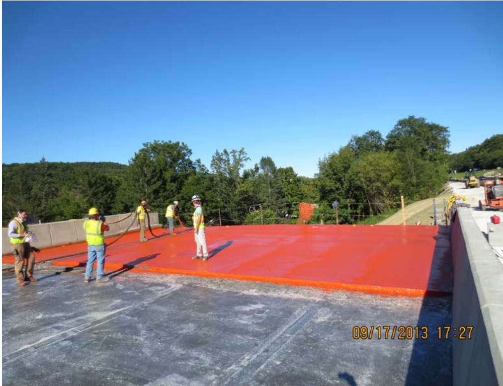
Figure 29. Photo. Placing the first layer of waterproofing membrane after priming the deck.
