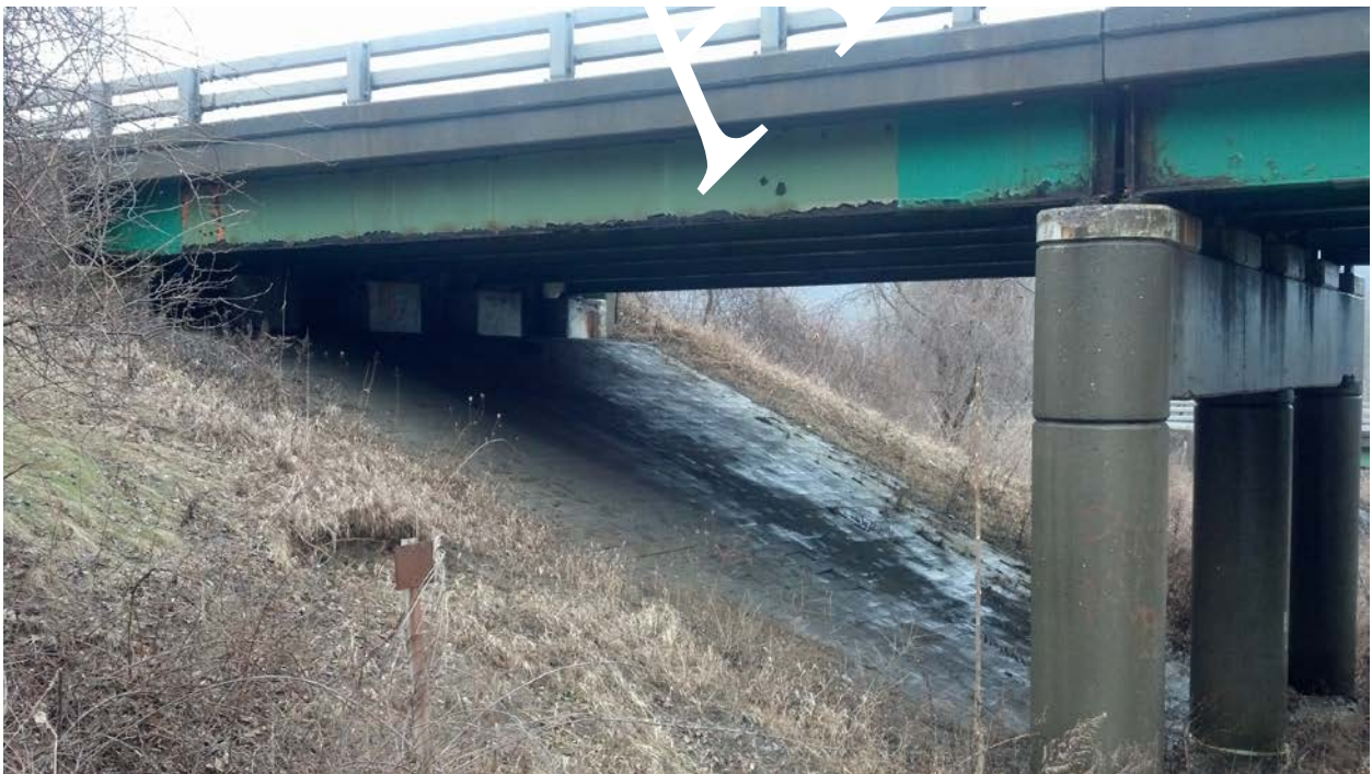
Figure 4. Photo. General deterioration of the girders.
