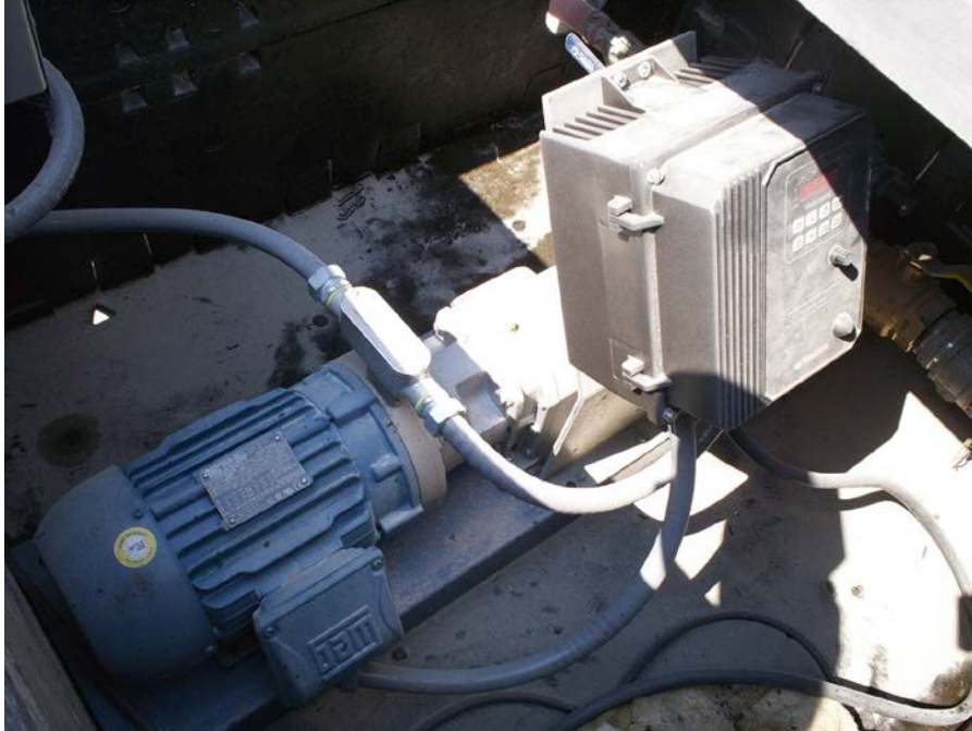
Figure 17. Photo. Additive pump. (courtesy: Wyoming DOT)
