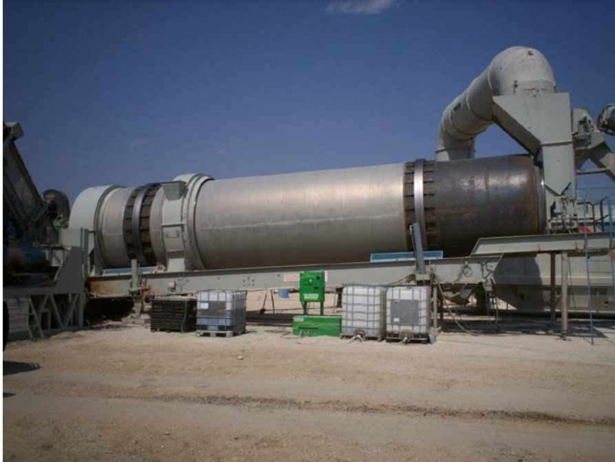
Figure 15. Photo. Gencor Ultra Drum 400 TPH, counterflow type. (courtesy: Wyoming DOT)
