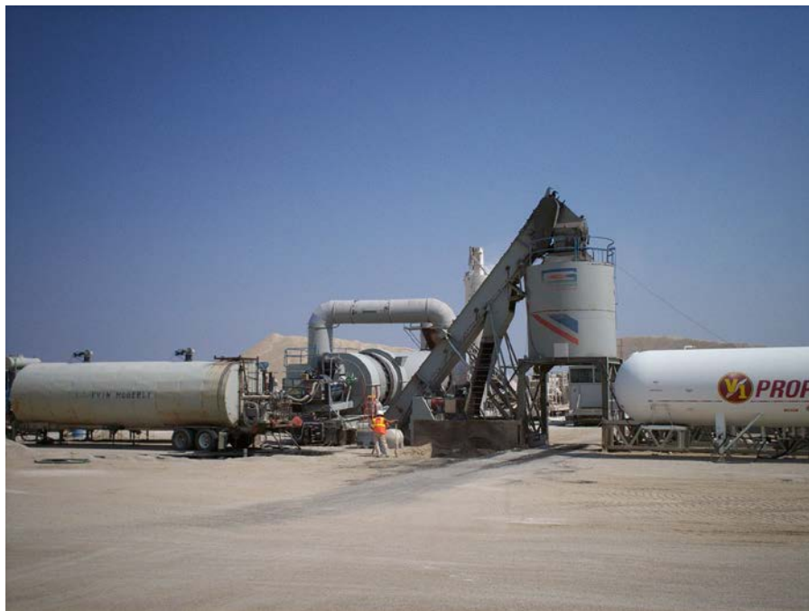
Figure 14. Photo. Gencor plant. (courtesy: Wyoming DOT)
