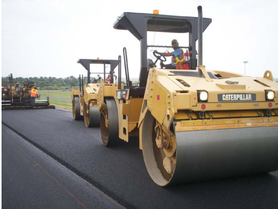
Figure 22. Photo. Steel rollers. (courtesy: Wyoming DOT)
