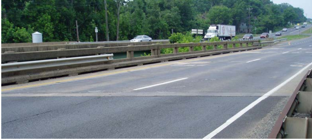
Figure 18. Prerehabilitated southbound bridge deck.
