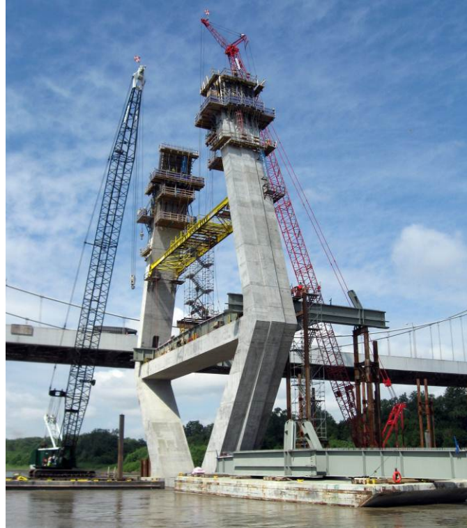
Figure 52. View of pylon construction and pier table placement from the river channel—August 2009.
