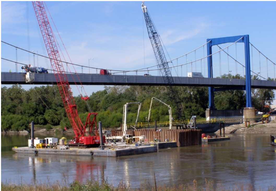
Figure 32. Placing 1,450 cubic ft of concrete in one day for the cofferdam seal—October 2008.
