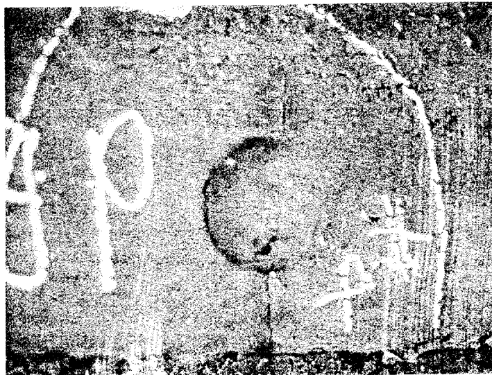
Obvious Cracking at a Rivet Hole
