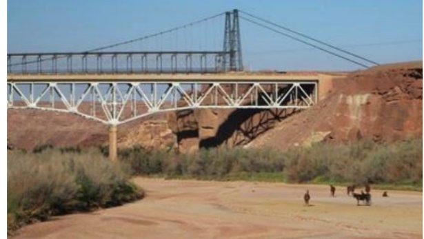
Figure 4: The U.S. 89 Bridge in Cameron, Arizona. (Image courtesy of Arizona Department of Transportation)
