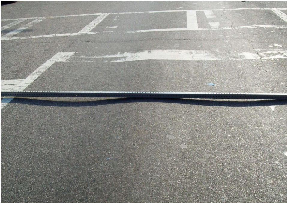
Figure 6. Photo. Existing pavement conditions.
