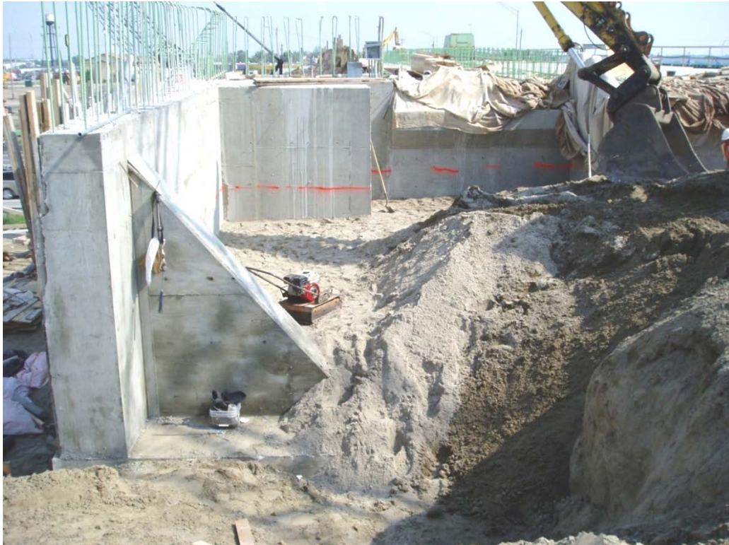
Figure 12. Granular material behind the abutment.
