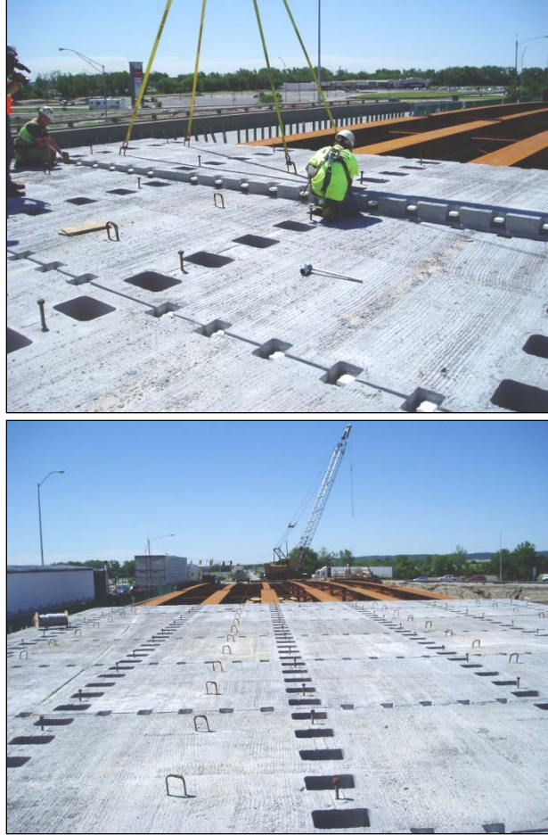
Figure 6. Panel being placed and several panels installed on the new bridge girders.
