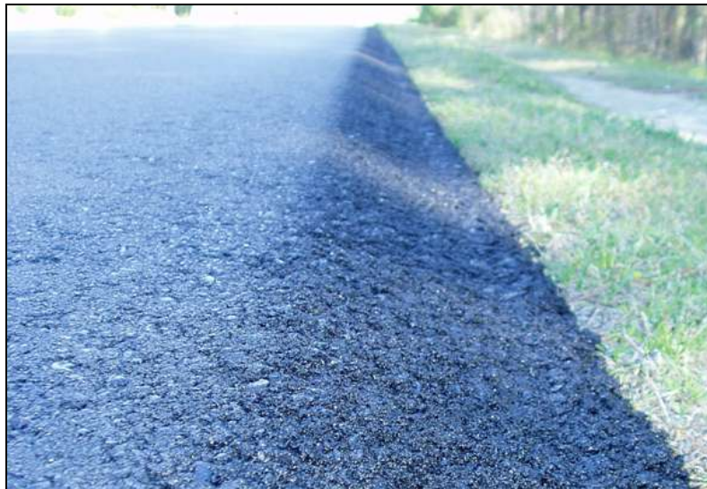
Figure 10. Texture of the Safety Edge SM slope face was nearly as smooth and sealed as the rest of the mat.
