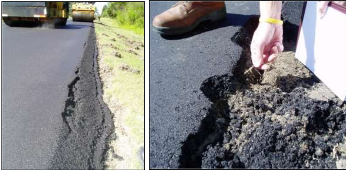
Figure 14. Isolated longitudinal edge cracking (left) and investigation revealed soil/vegetation under the pavement edge (right).
