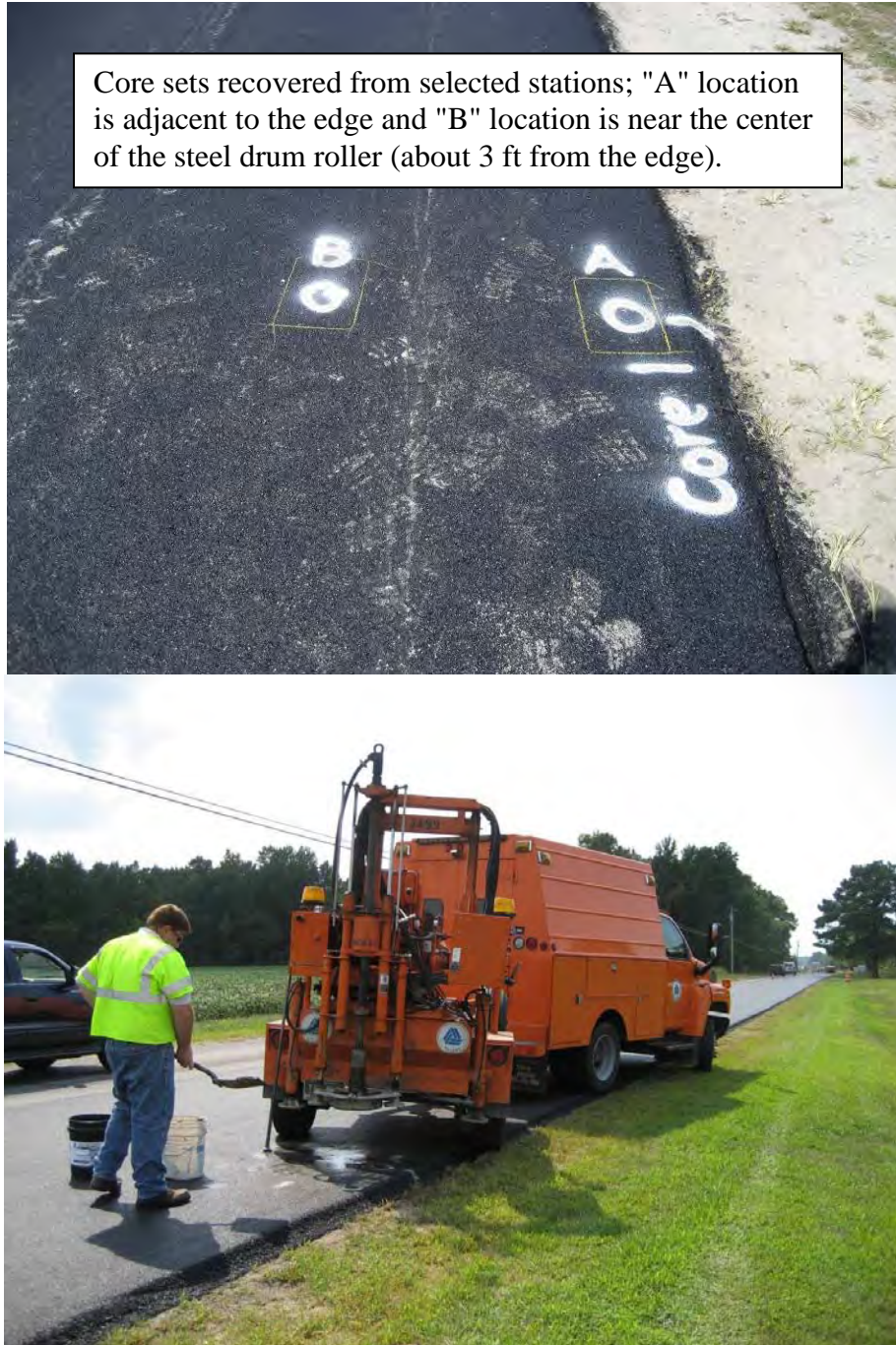
Figure 10. Photos showing location of cores and nuclear density tests made with the Troxler 3430 gauge (nuclear density readings were taken and then the WMA mix was cored).
