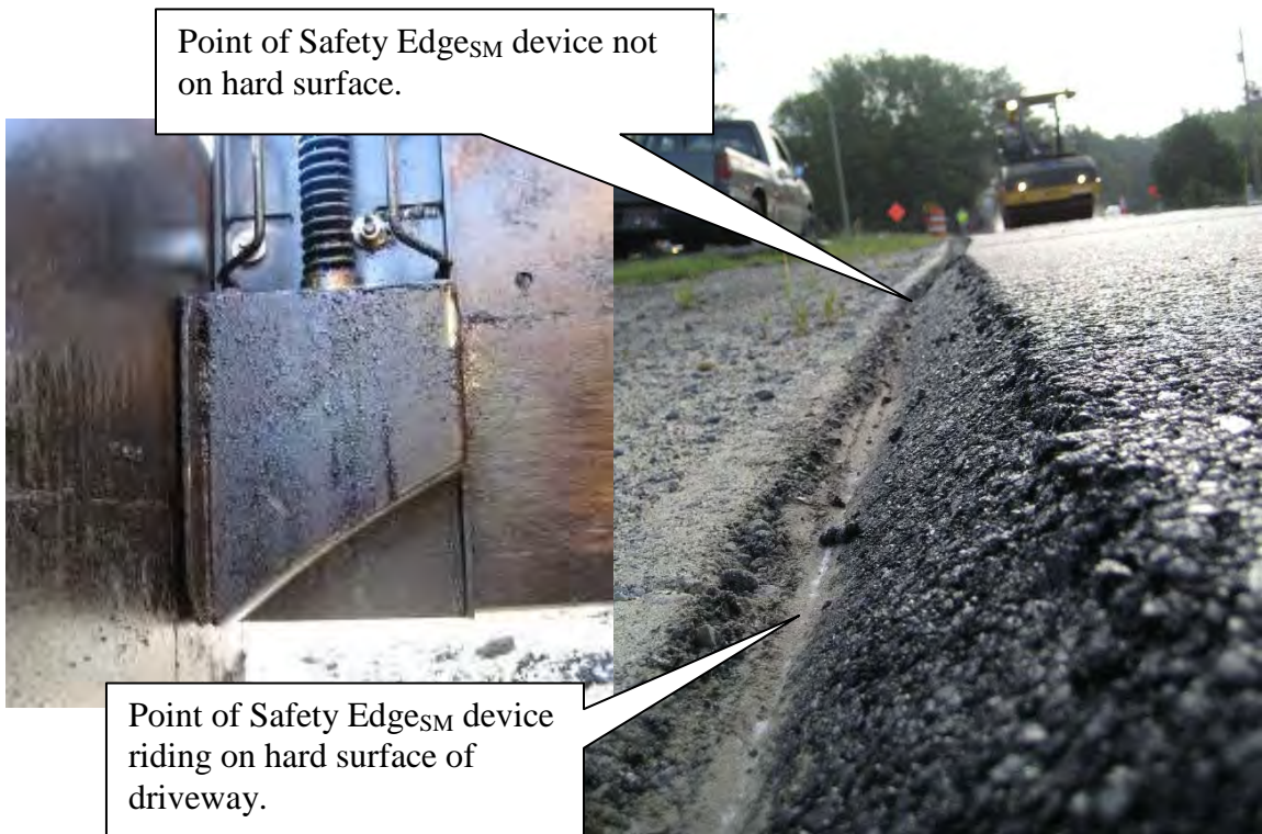
Figure 18. Point of Safety Edge SM scratching the surface of an intersecting driveway.
