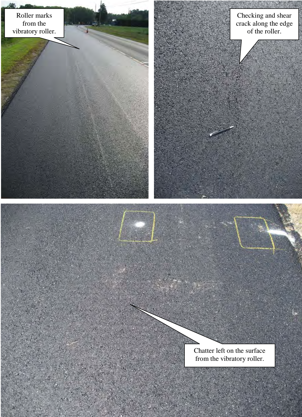
Figure 22. Surface defects observed after rolling.
