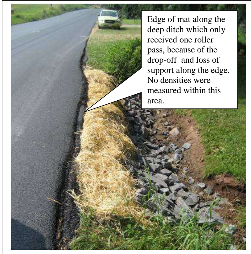
Figure 3. Localized area with deep ditches adjacent to the pavement.
