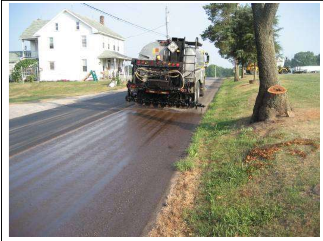
Figure 15. An emulsion was used as a tack coat prior to HMA placement (note the material that was added to the edge of the pavement to widen the roadway).
