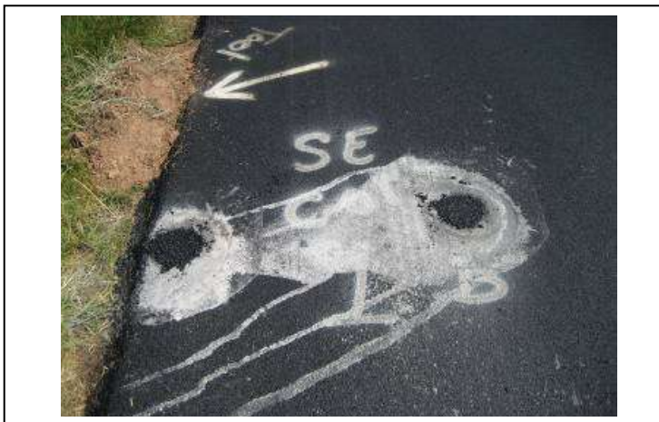
Core #1; Safety Edge SM section (A location is adjacent to the Edge; B location is near the center of the steel drum roller (about 3 feet from edge).
