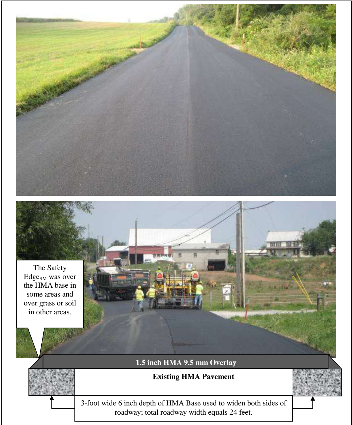
Figure 2. General overview of the 1.5 inch HMA layer placed along the project and pavement cross section provided by the Pennsylvania DOT.
