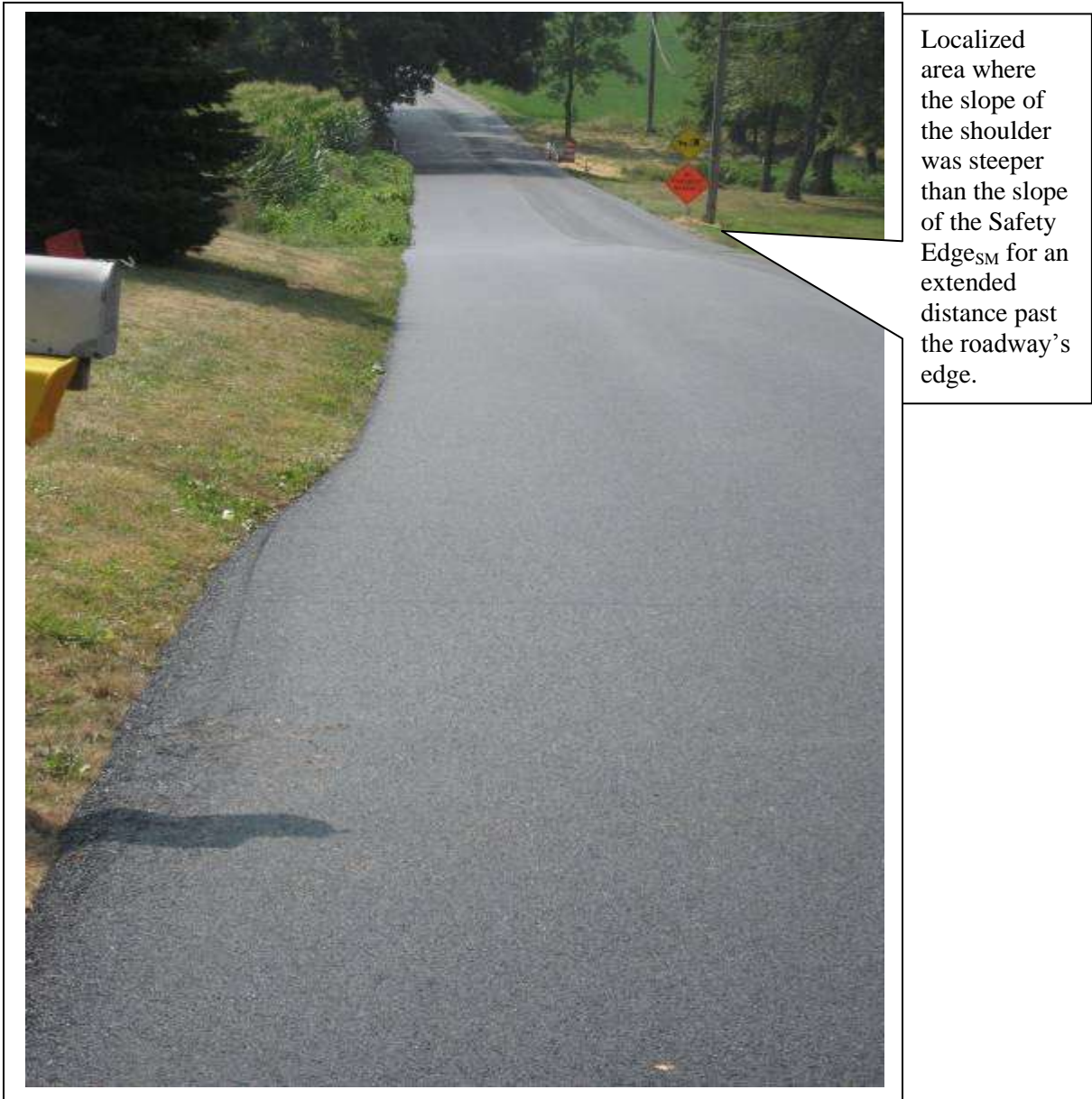
Figure 19. Area where the slope of the shoulder was steeper than the Safety Edge SM slope.
