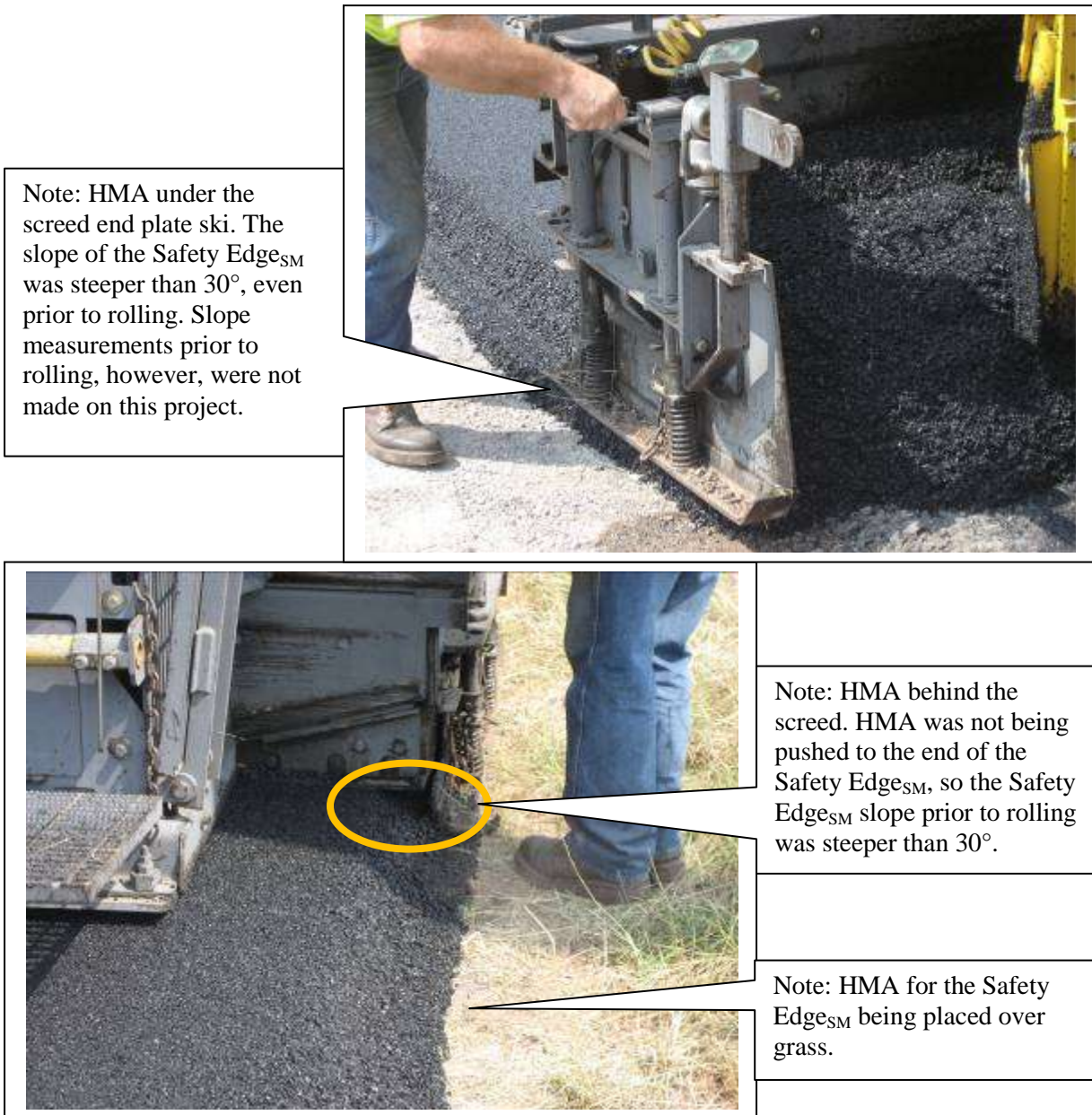
Figure 23. HMA shown under and behind the screed; the HMA was not pushed to the end of the Safety Edge SM resulting in a steeper slope prior to rolling.
