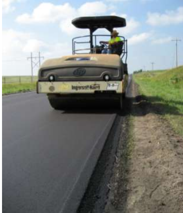
Figure 21. First pass of the Ingersoll-Rand finish roller along the Safety Edge SM .
