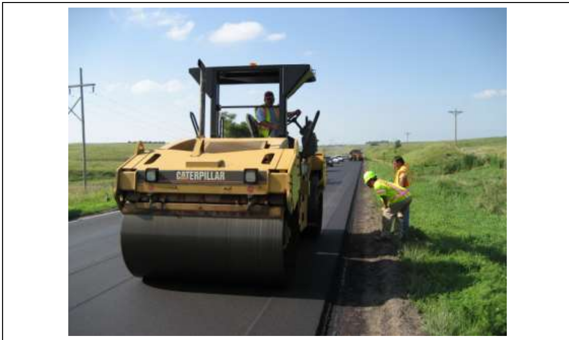
Pass #3 of Caterpillar roller is 6 to 12 inches from the edge of the mat.
