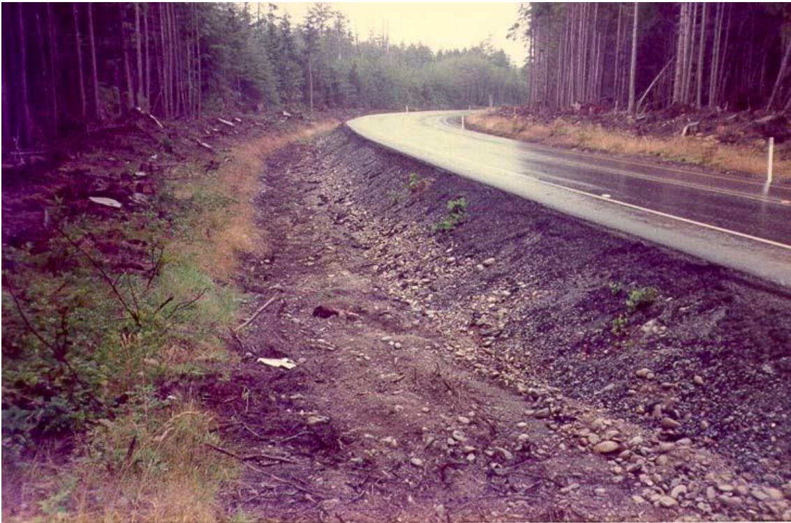
Figure 2. Example of where a foreslope/embankment is too steep for the Safety Edges SM .
