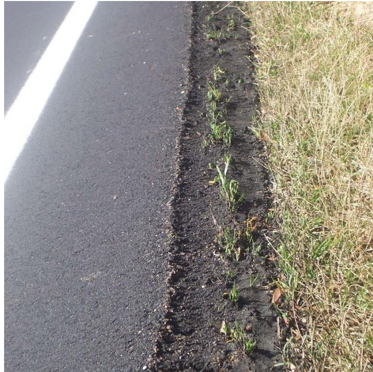
Figure 6. Example of Safety Edges SM placed on heavy vegetation – due to lack of adequate compaction the Safety Edges SM will deteriorate.
