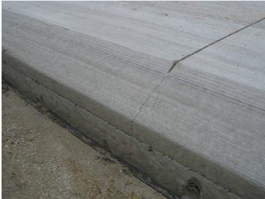
Figure 16. Sawcut and crack at the formed joint on one of the Safety Edges SM demonstration projects.
