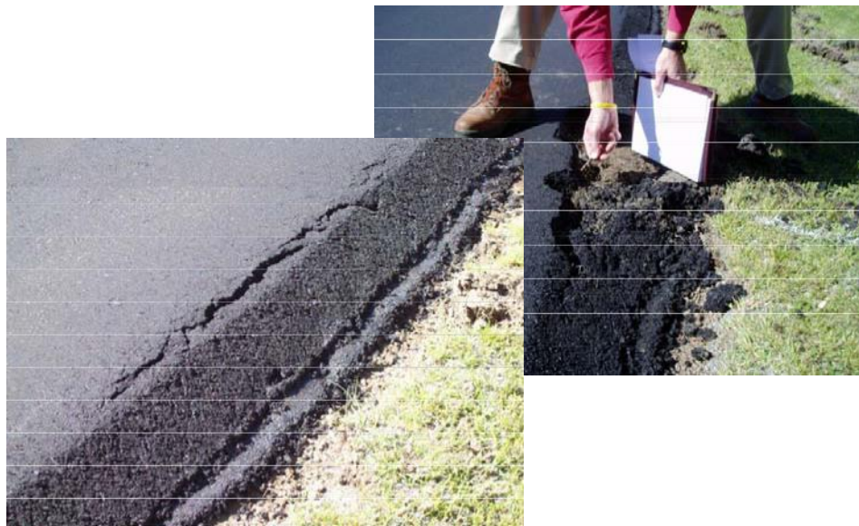
Figure 11. Longitudinal crack due to Safety Edges SM break point located on unimproved shoulder.
