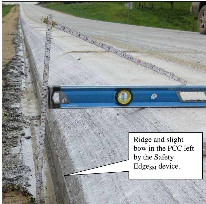
Figure 5. Slope face showing ridge and bow.
