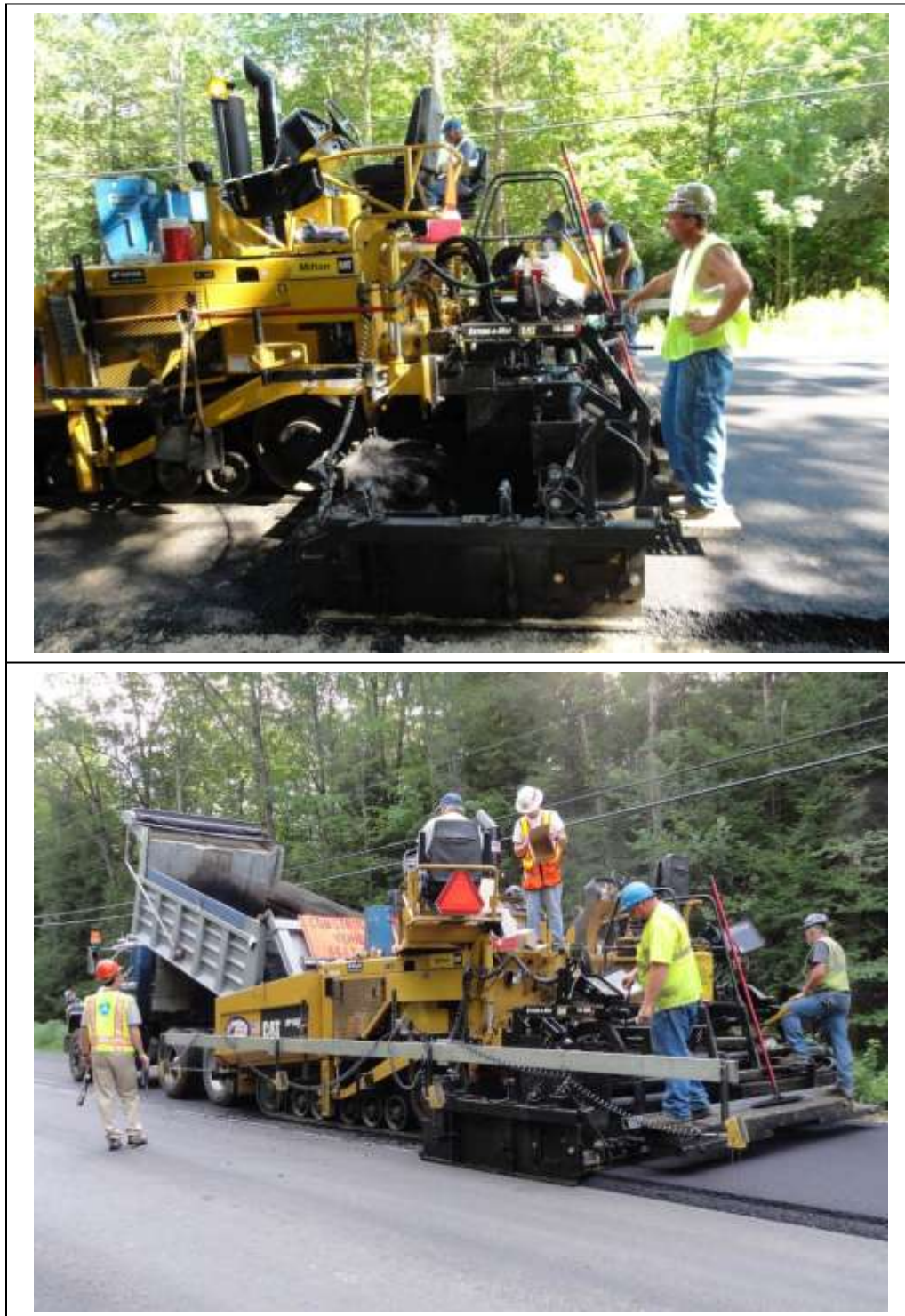
Figure 18. Paving operations showing the Safety Edges SM paved using the Advant-Edger and the centerline joint paved using the TransTech Notched Wedge Joint Maker.
