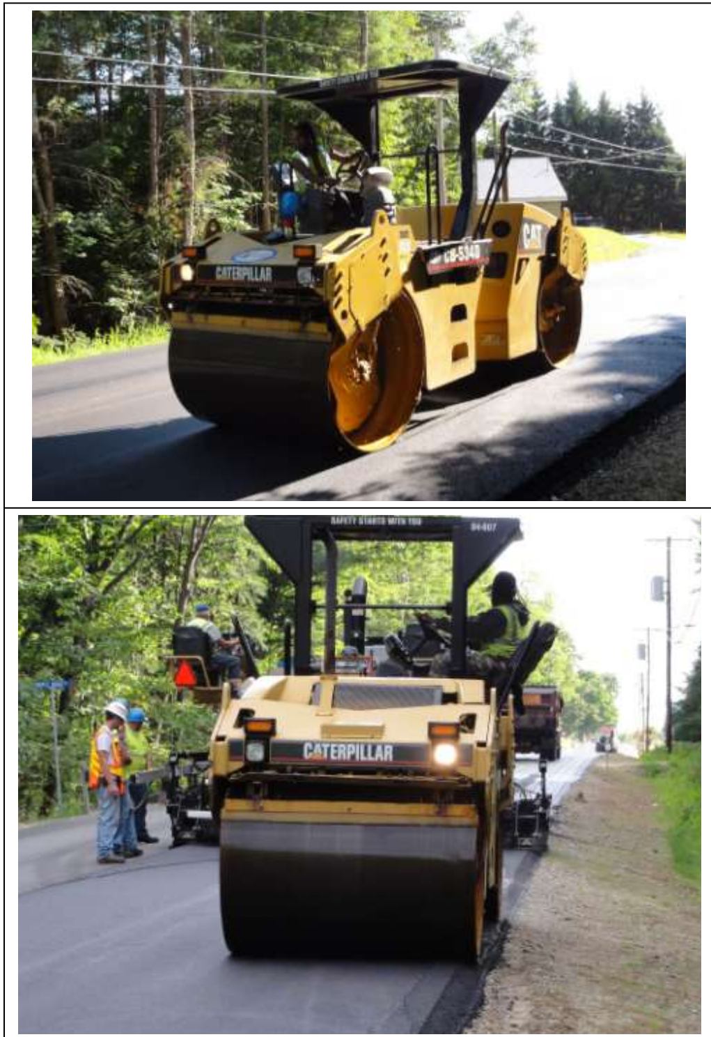
Figure 20. Steel wheel roller used in the breakdown position to compact the 12.5 mm HMA mix.
