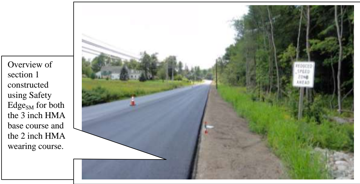
Figure 4. General overview showing the wearing course with Safety Edge SM . Image taken facing the southbound direction around station 374+53, the end of section 1.
