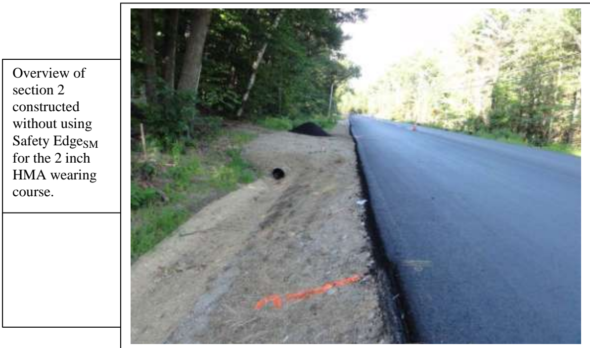
Figure 5. General overview showing the wearing course without Safety Edge SM . Image taken facing the northbound direction around station 385+38, the beginning of section 2.
