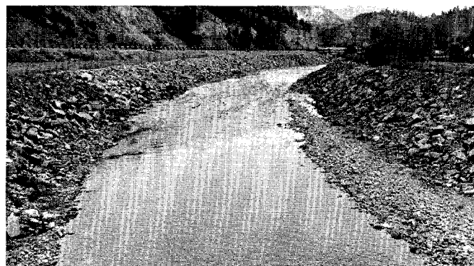
Figure 67. View downstream, from Main Street bridge, along relocated channel of Pine Creek. Erosion during 1974 flood occurred along bank in left background.
