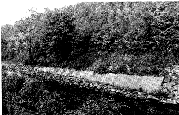
Figure 178. View upstream along Shamokin Creek, showing bank slumping above remaining concrete slope pavement, and rock riprap installed in 1972.
