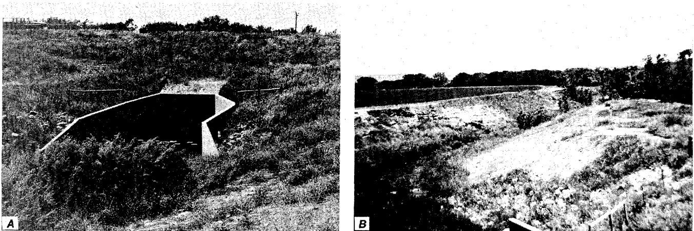
Figure 151. One Mile Creek at site 72. A, Culvert and stilling basin at downstream side of roadway embankment. B, View downstream from bridge along relocated channel of One Mile Creek, in 1979.
