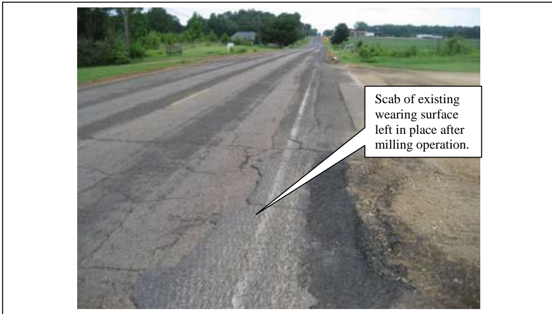
Figure 3. General overview of the existing HMA pavement after milling; heavily distressed area with cracking (view is towards the east).
