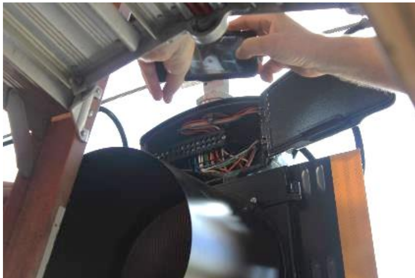
Figure 43: Disconnect box for 3-section signal with no visible damage
