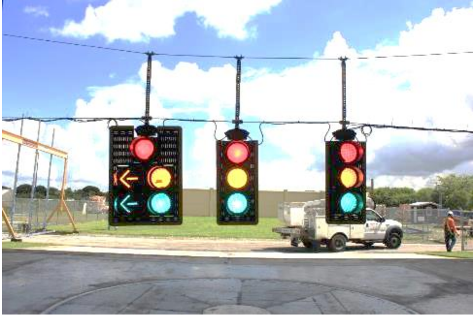
Figure 28: Signal assemblies installed on test rig (before testing)
