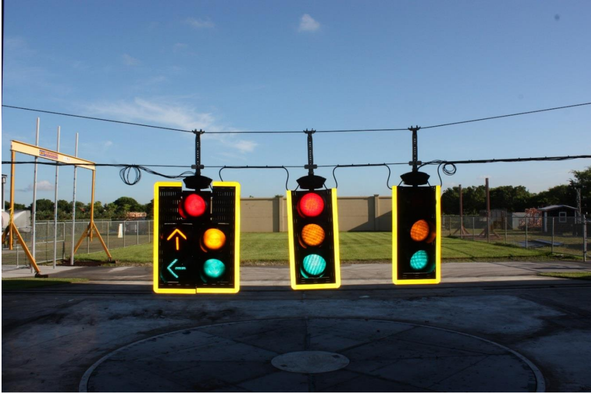
Figure 90: Signal assemblies installed on test rig (before testing)
