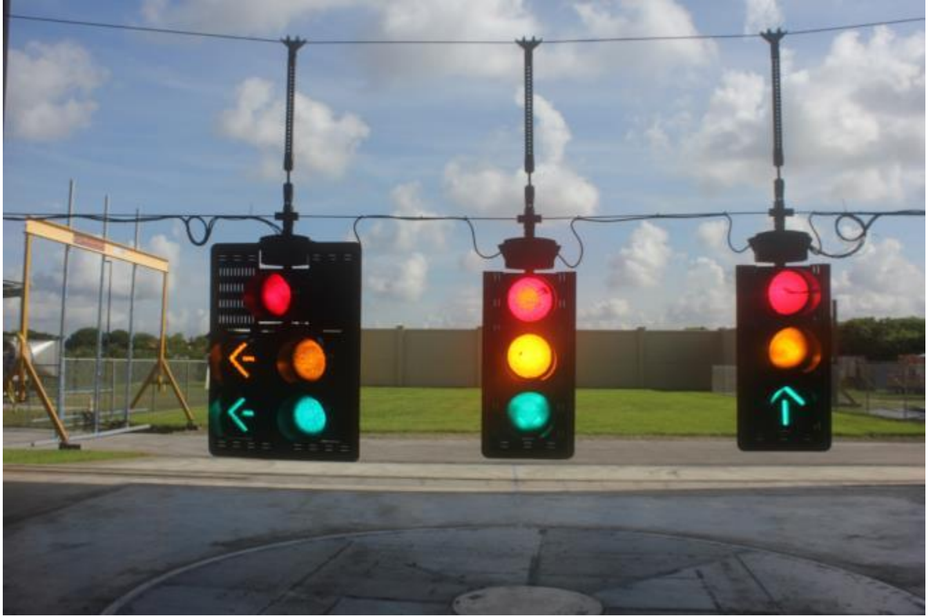
Figure 59: Signal assemblies installed on test rig (before testing)
