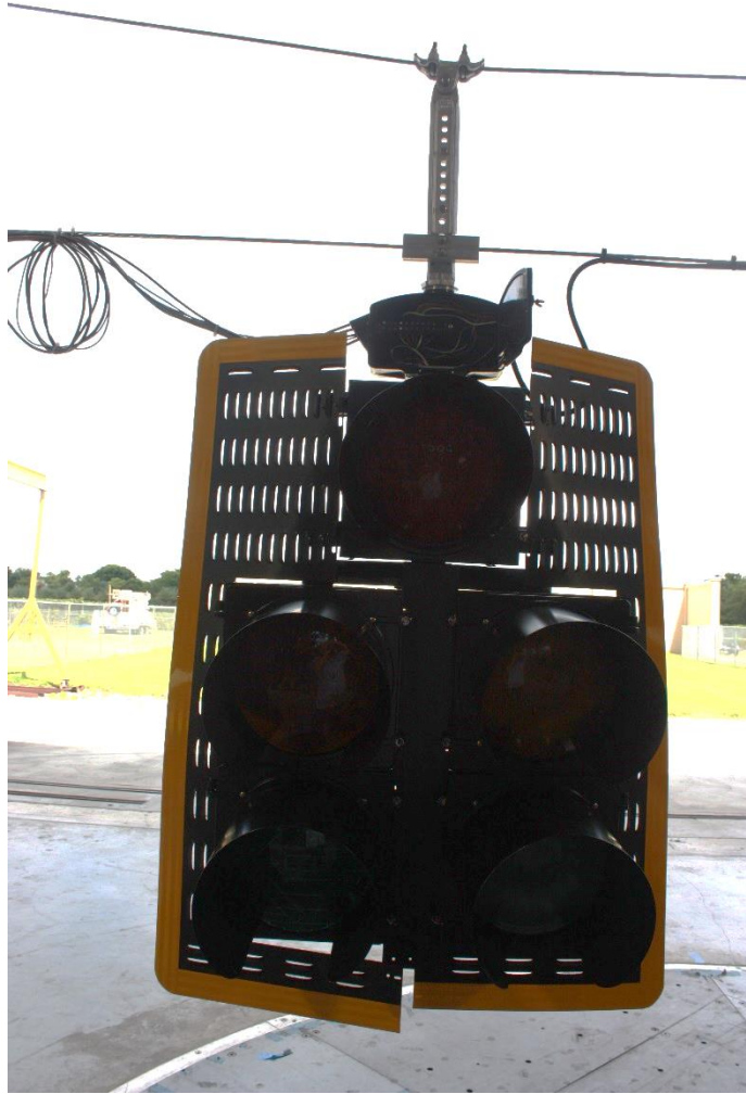
Figure 102: 5-Section signal with damaged back plates
