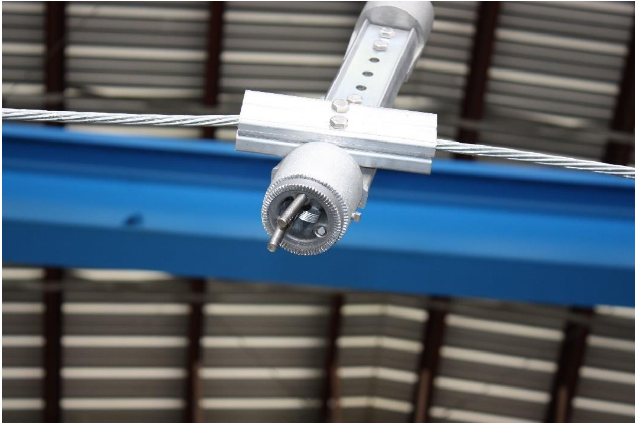
Figure 131: Adjustable hanger to disconnect box connection failure (5-section assembly)
