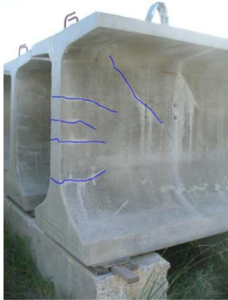
Figure 2-3 End zone cracks, marked in blue (Hamilton et al. 2013)
