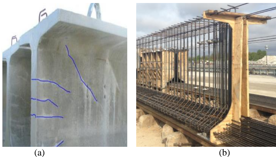
Figure 1-1 End region cracking (a) (highlighted in blue) (Hamilton et al. 2013) and conventional end region reinforcement (b)
