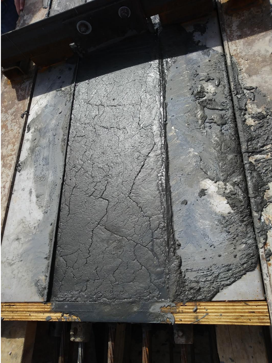
Figure 2-16: Plastic shrinkage cracking formed approximately 20 minutes after UHPC placement
