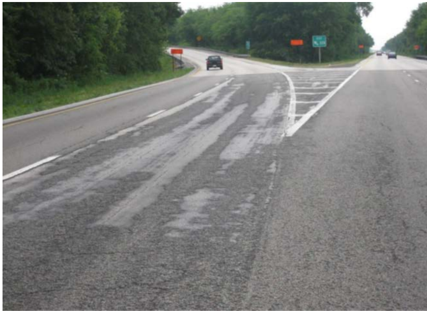
Figure 1. Raveling of One Florida OGFC Project (Bennert and Cooley, 2014)
