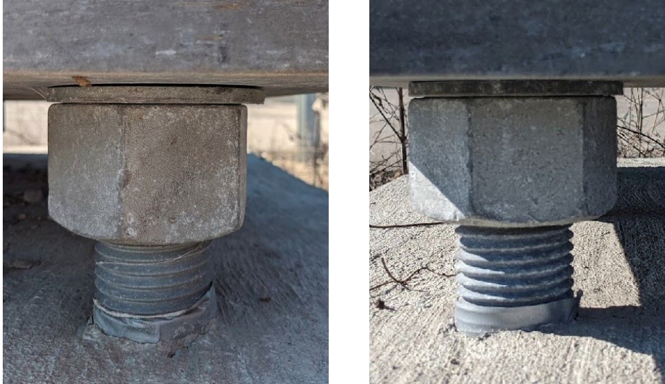
Figure 3.2.7 Gap between baseplate and washer #5 out of plumb (left) and bolt #8 plumb for reference (right)
