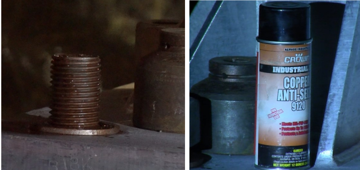
Figure 3.2.3 Lubricated anchor rod connection (left) and lubricant utilized (right)
