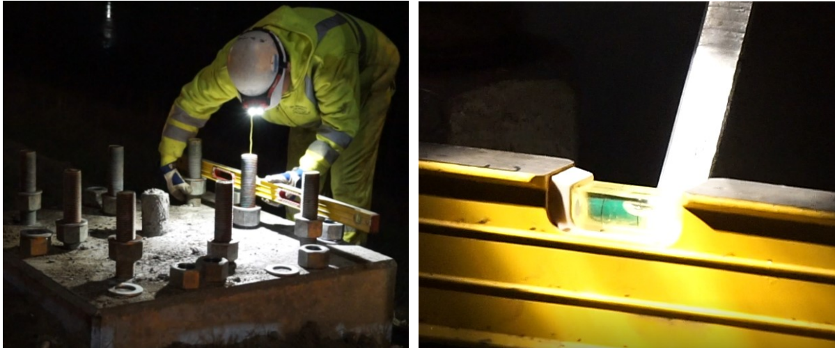
Figure 3.2.2 Leveling nuts on sign truss structure (left) and final installation of COSS out of plumb (right)
