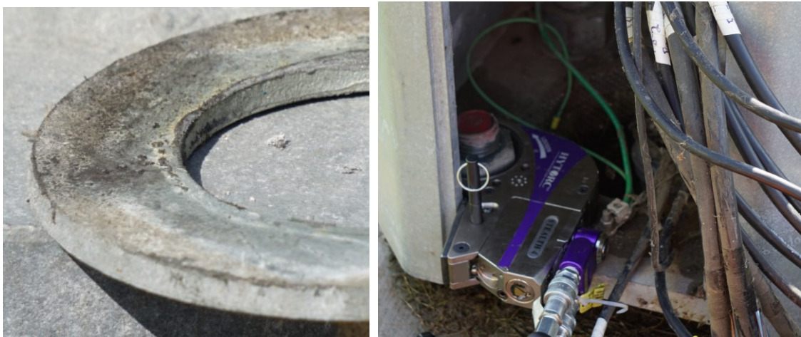
Figure 3.3.13 Galvanizing dimples on washer (left) and moved grounding wire (right)
