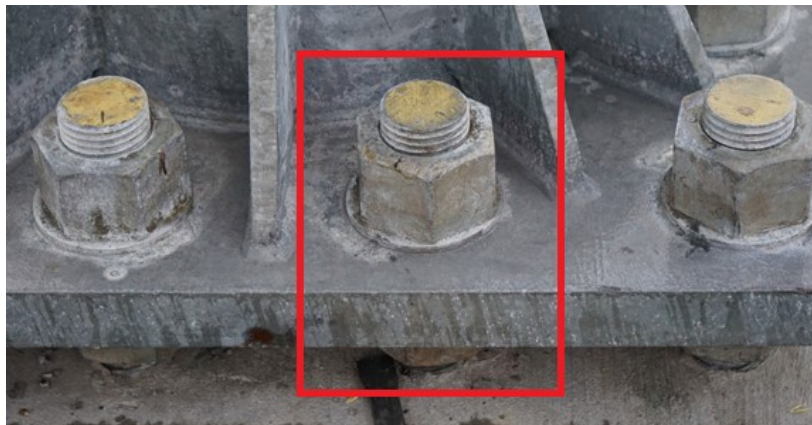
Figure 3.2.6 Out-of-plumb anchor rod on COSS OH 280-023
