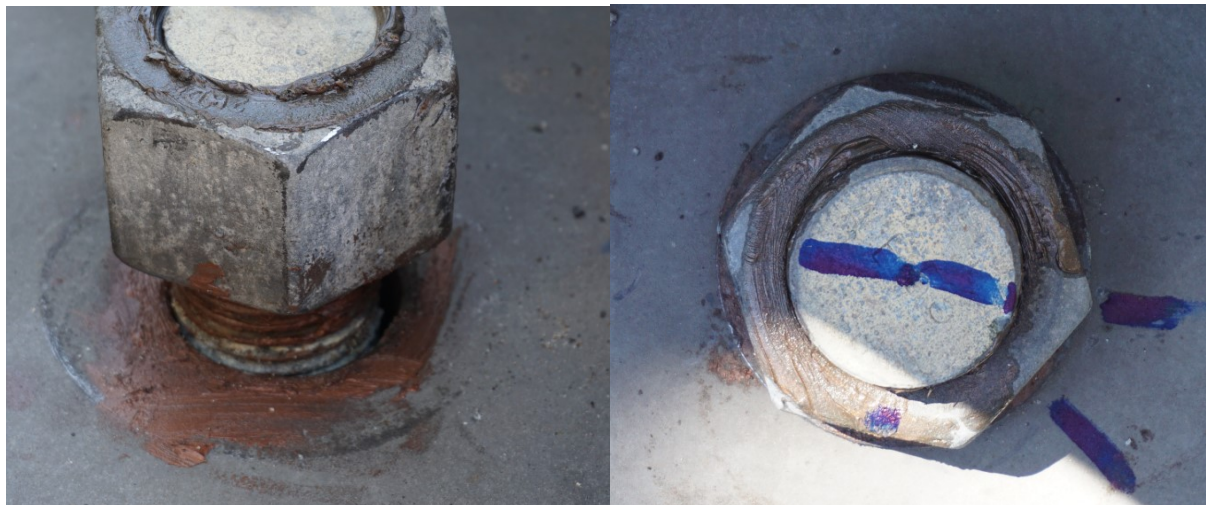
Figure 3.2.15 Missing washer on rod 8 (left) and excessive turn of nut on rod 11 (right)
