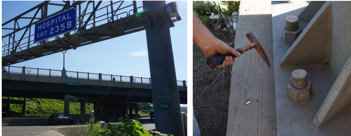
Figure 3.2.11 Full truss OH sign I-94-602 (left) and inspecting rod pre-tension force (right)
