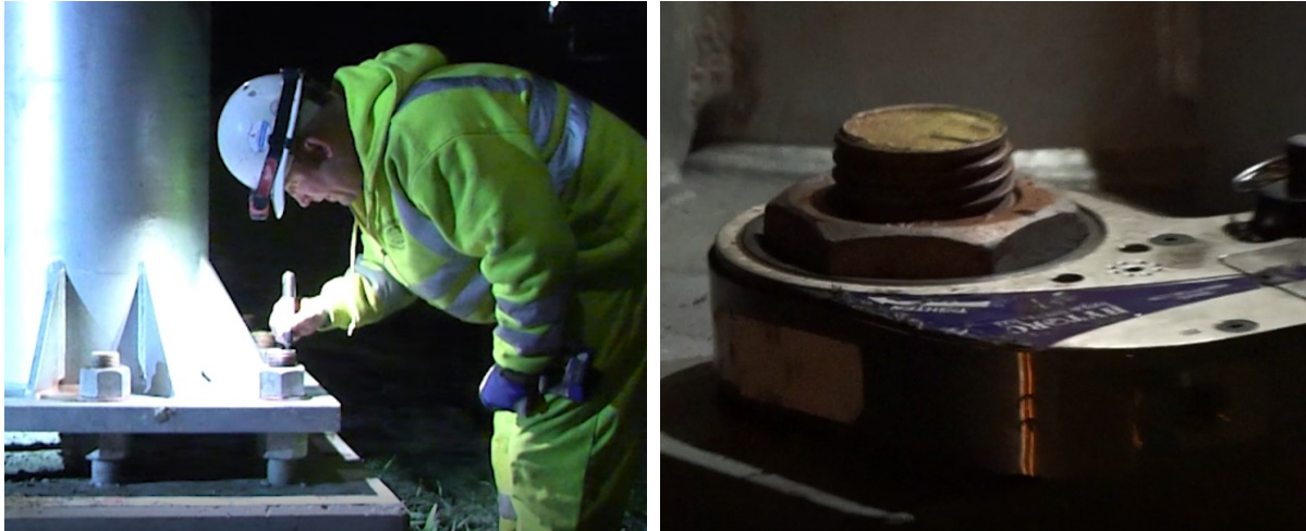
Figure 3.2.5 Marking each rod and nut as reference for the turn-of-nut tightening (left) and tightening using a hydraulic wrench (right)
