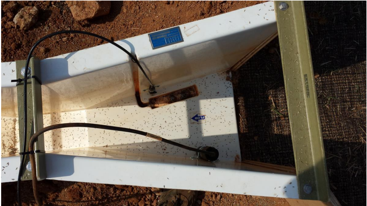
Figure B.7. Probes mounted in the 6" Parshall Flume.
