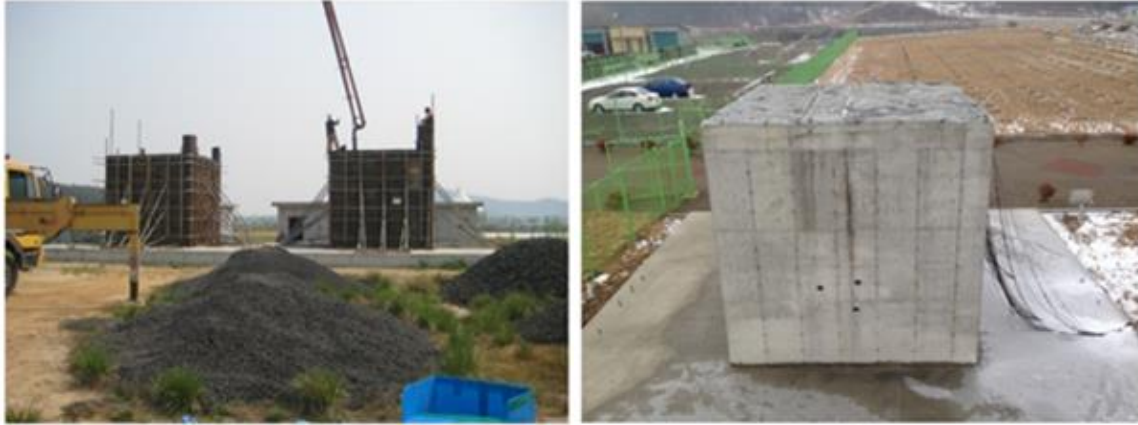
(a) concrete casting in the field (b) mock-up test member in field testing
