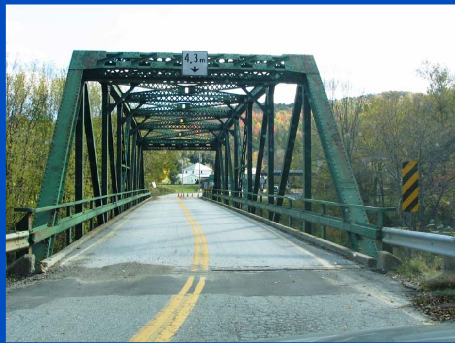
The bridge pictured above is the Sutton—East Richford Bridge. Collaboration between Québec's MTQ and Vermont's VTrans to reconstruct this bridge were discussed during the November 17th meeting.
