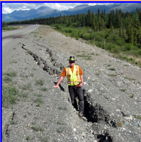
Paul Murchison, Director, Yukon Highways and Public Works, stands in a crack along the Alaska highway caused by permafrost
