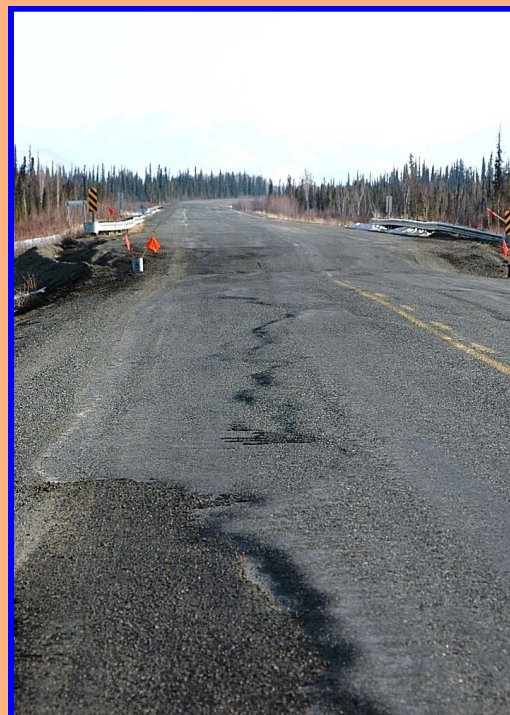
A photograph of the highway distortions caused by permafrost
