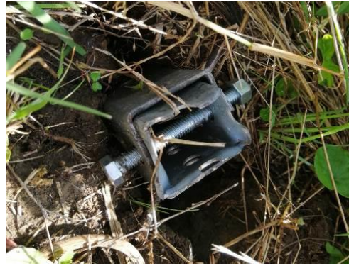
(b) Traffic Sign 2000 Main Body Broken
