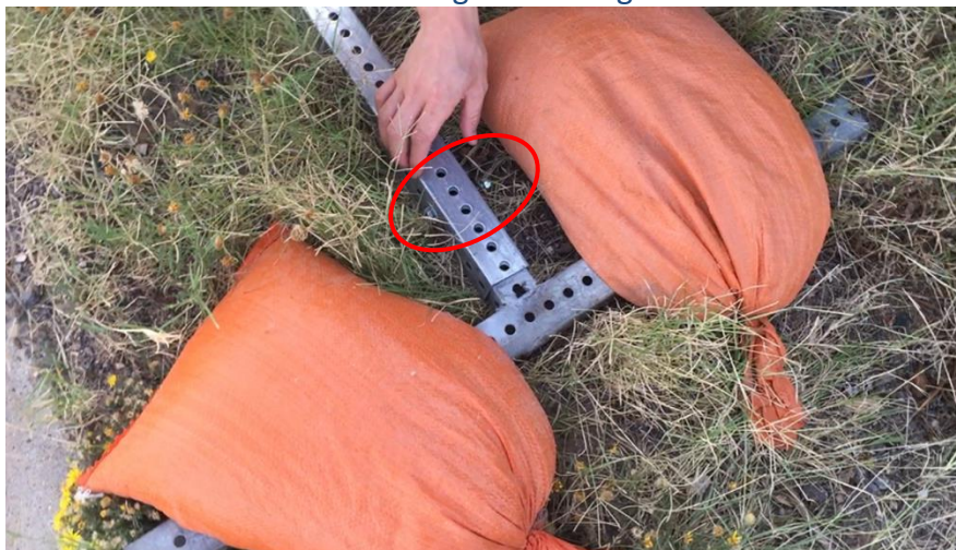
b. The loosened nut resulted from the constant trembling of the supported traffic sign Figure 50. Performance Checks of Traffic Signs in Midland, TX
