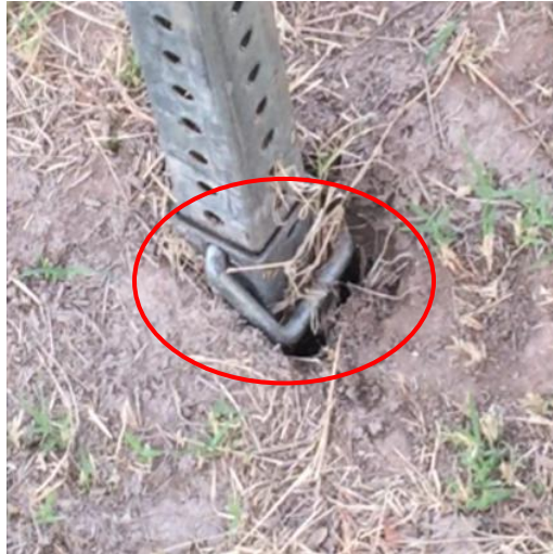
a. The hole (the gap between the metal post and the earth) caused by the constant traffic sign trembling
