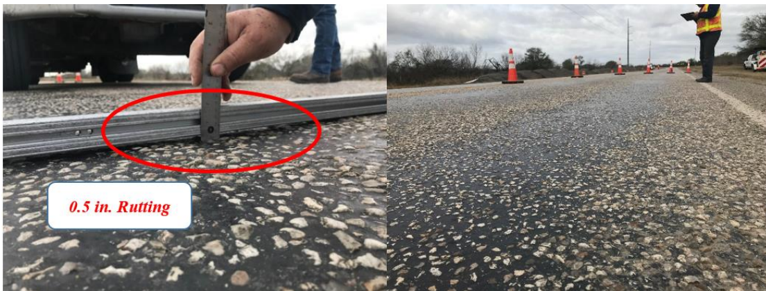
Figure 7.5. Rutting Measurements in FM 468, Laredo District.
