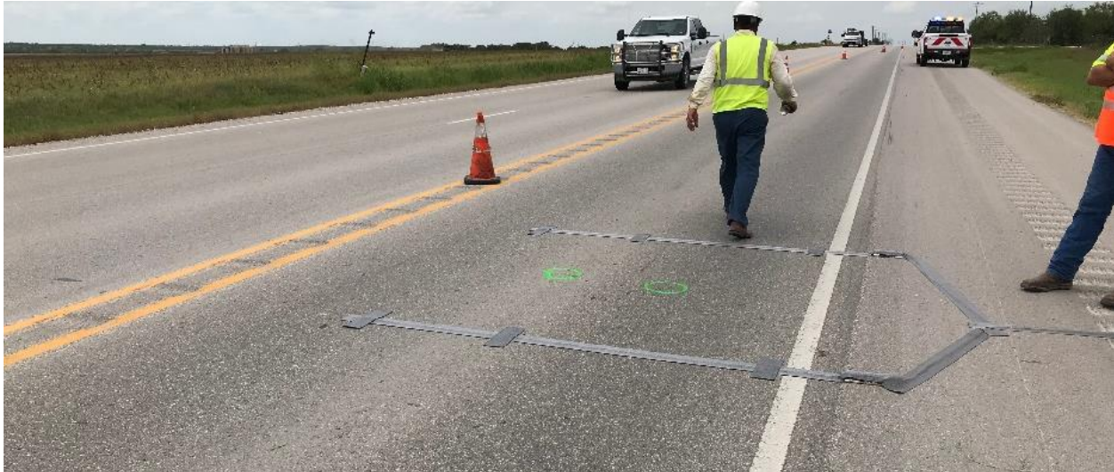
Figure A.15. Pavement Conditions of SH 72 –Karnes County
