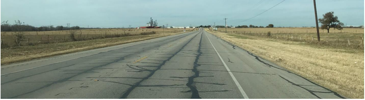
Figure A.20. Longitudinal Cracks of US 183 - Gonzales County
