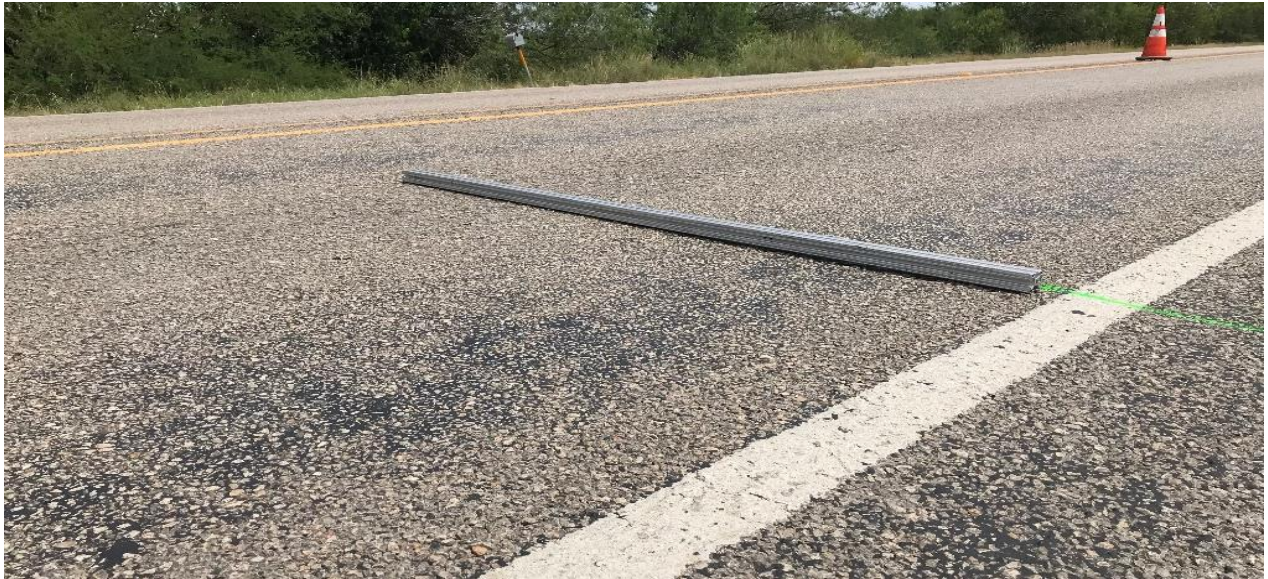
Figure A.16. Shallow Rutting in BU 181/SH 123 –Karnes County
