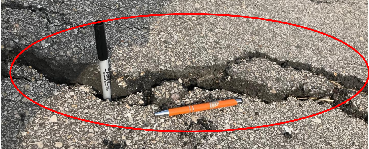
Figure A.14. Longitudinal Cracking in Right Shoulder in US 281 –Live Oak County
