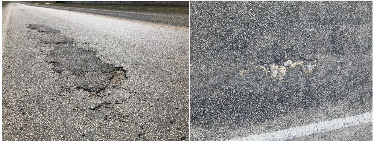
Figure A.9. Pothole Formation in FM 99 - McMullen County
