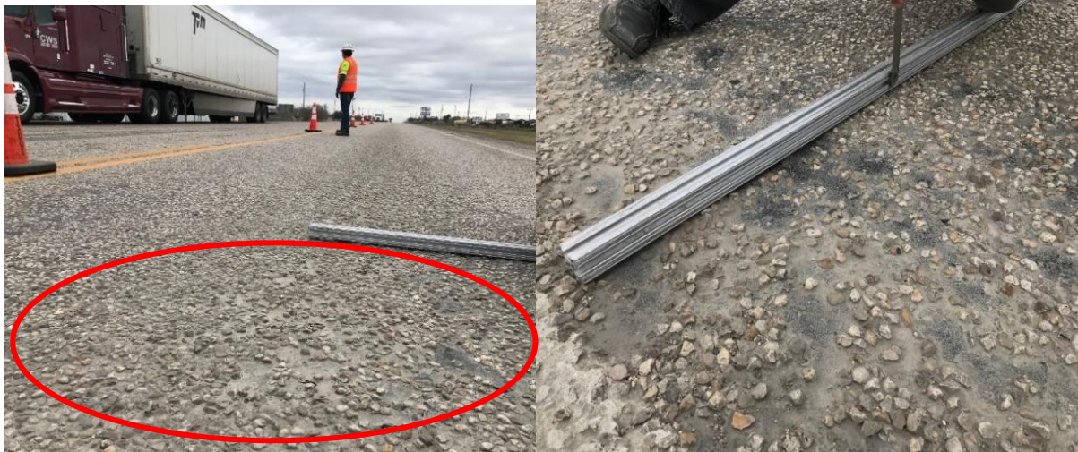
Figure A.4. Raveling and Missing Aggregate in US 83 -Dimmit County
