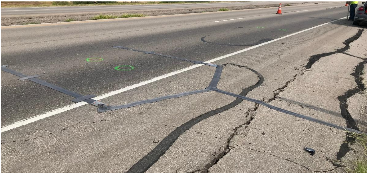
Figure A.13. Longitudinal Cracks in US 281 – Live Oak County
