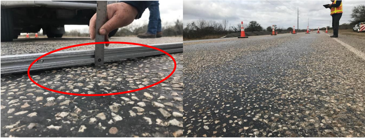
Figure A.2. Shallow Rutting in FM 468 - La Salle County
