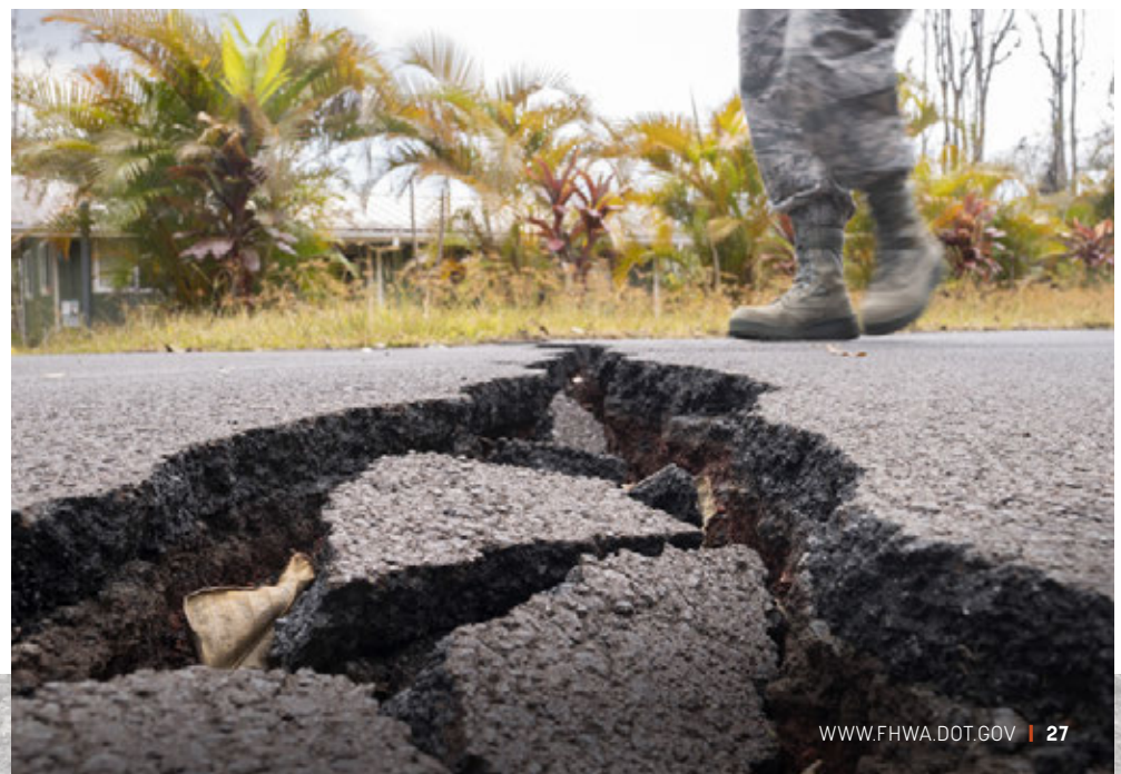
A Hawaii Air National Guard Airman approaches a growing road crack during a volcanic outbreak at Leilani Estates in May 2018.
