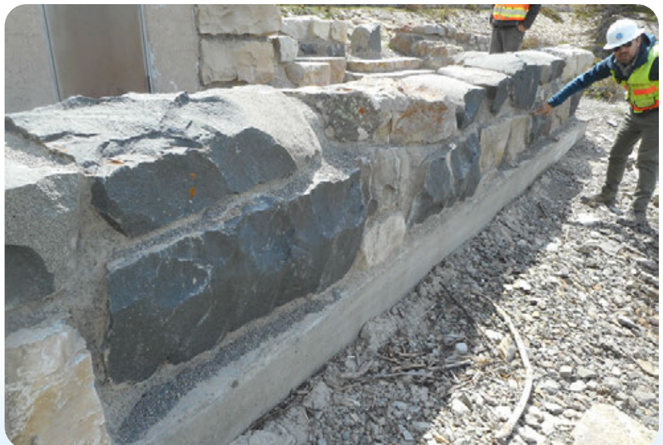
Along most of Going-to-the-Sun Road, existing rails and border walls needed repair. Here, a worker inspects a completed section of wall.
