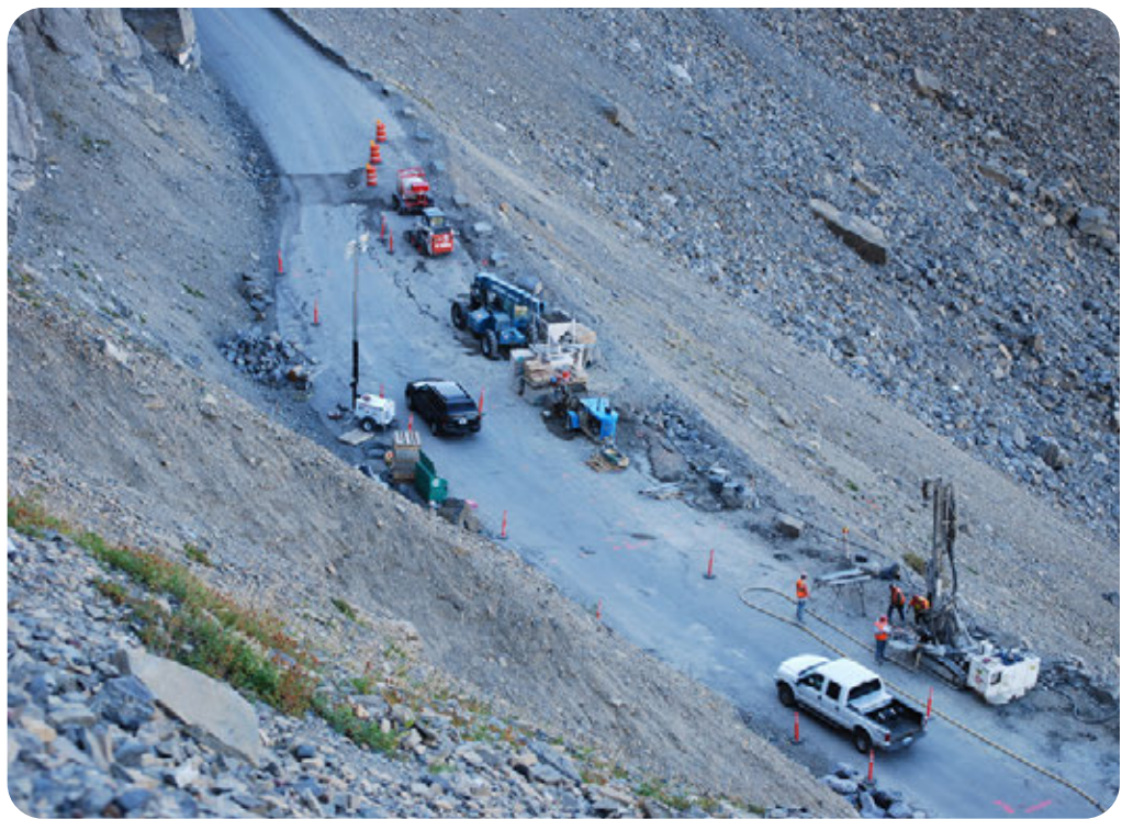
Crews had to mitigate rockfall risks and support rock faces along the road while maintaining the natural look of the surrounding area.
