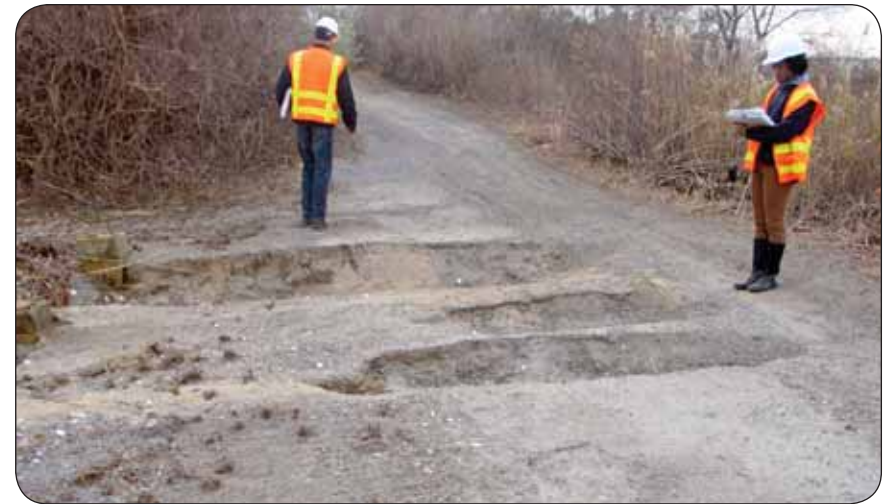
Damage inspection on refuge road, Jamaica Bay, Long Island, New York
