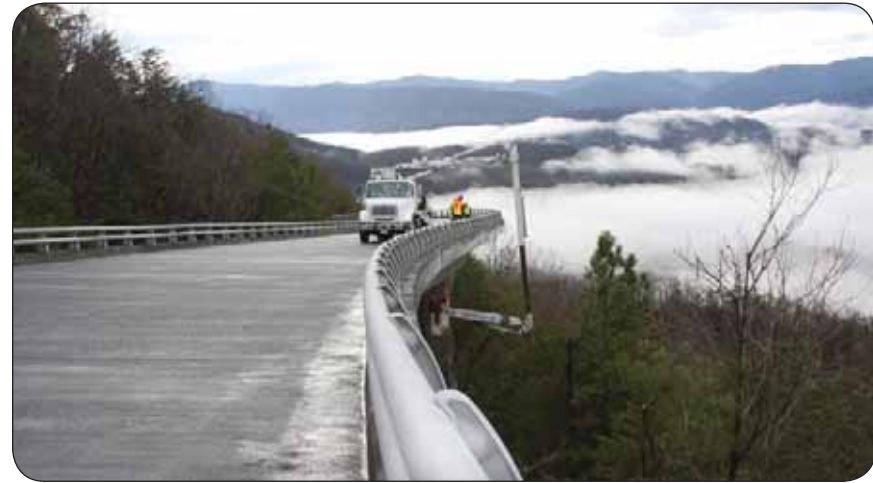
FLH Bridge Inspection Vehicle the "Snooper" inspecting a newly completed section of Foothills Parkway Bridge 2 — Great Smoky Mountains National Park, Tennessee
