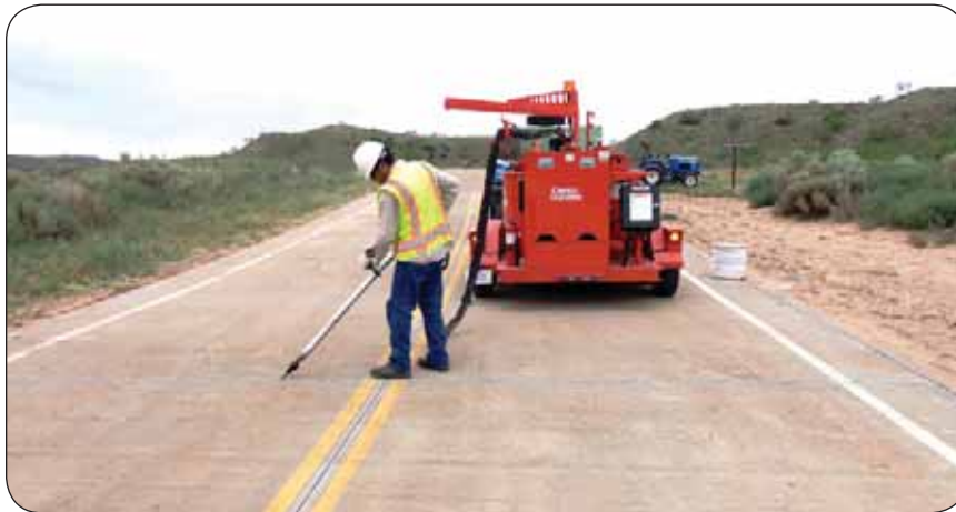
Pavement Preservation Program — joint cleaning and resealing on portland cement concrete pavement (PCCP) — Lake Meredith National Recreation Area, Texas
