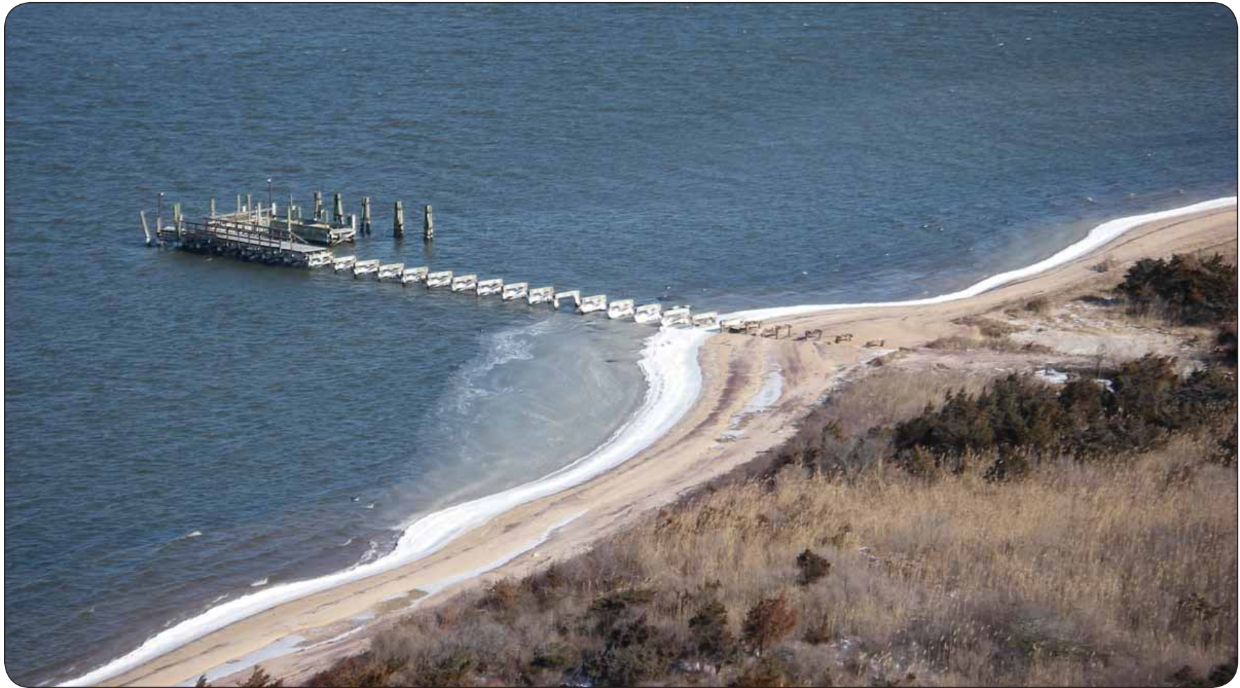
View of damaged visitor use dock near Fire Island Lighthouse, Great South Bay, Long Island, New York
