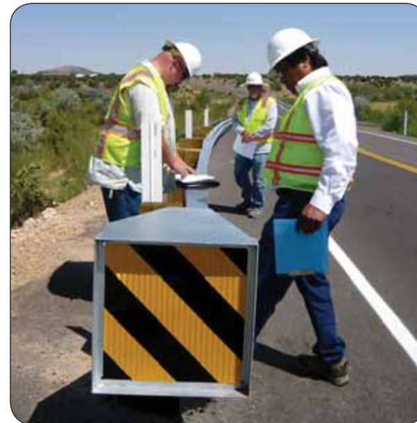
Safety measures included installation of guardrail — Acoma Pueblo Transportation Director (right foreground) performing an inspection
