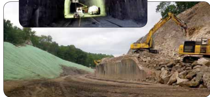
Example of an open cut tunnel, full excavation of rock and soil from the top of the tunnel, fully exposing the track, creating a valley. A portion of the original brick lining of the tunnel wall is visible on the right — Shoofly Tunnel near Markelton, Pennsylvania
