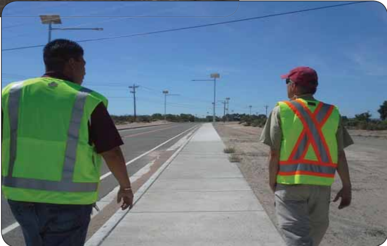
After — Ohkay Owingeh Public Works Director accompanies FHWA personnel during Final Inspection tour of the new all-weather surfaced road which now includes sidewalk, curb, gutter and solar lighting.
