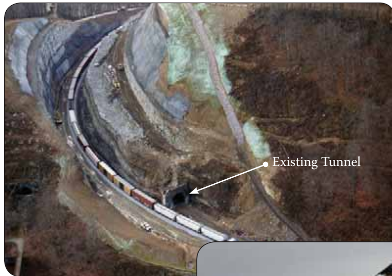
Train traffic continues to travel through the Pinkerton Tunnel Run-Around-Track while construction is underway to remove the existing tunnel. — Markelton, Pennsylvania
