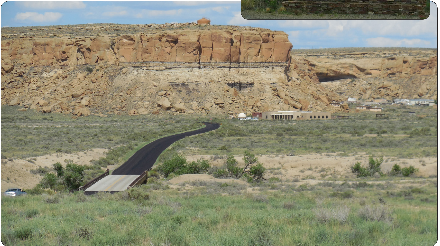
Chaco Culture National Historical Park, Visitors Center Access Road and Bridge Reconstruction, New Mexico
