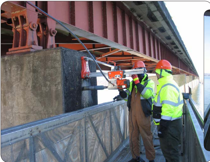
Horizontal Concrete Coring or Concrete Core Drilling performed by FLH Bridge Inspection staff as part of the in-depth investigation into the condition of bridge piers on the John Coffey Bridge. The retrieved concrete samples were laboratory tested to evaluate the concrete and verify initial bridge inspection findings.
