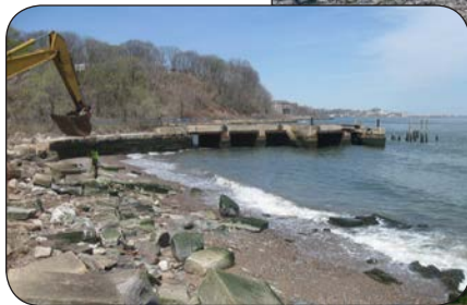
Major Breach Area, Historic Boat Dock
