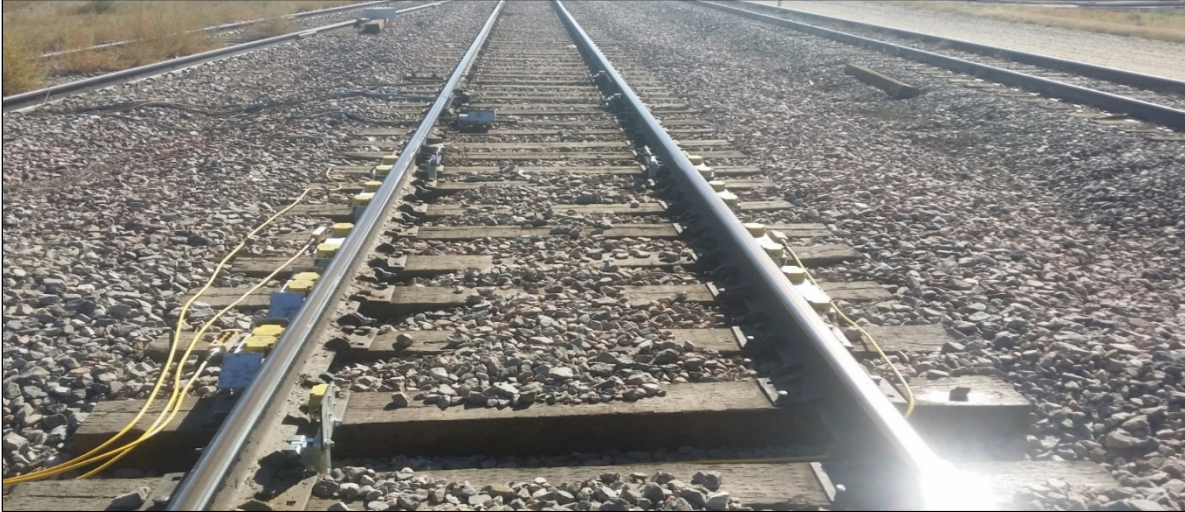
Figure 14. Broken Rim Detector System Installed at the TTC
