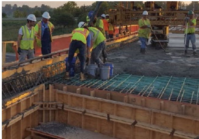
Figure 1-1 – Field implementation of flowable FRC with adapted rheology for construction of a bridge deck near Taos, Missouri
