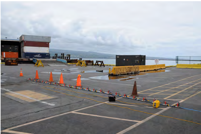
Figure 9. SR surveying at Hilo Harbor (note settlement depressions in asphalt pavement)
