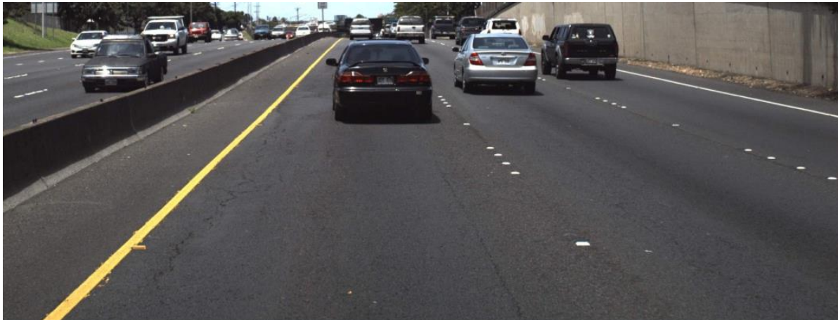
Figure 7-4. Example of left lane with more deterioration than the rightmost lane (Route H-1, MP- 21.027).
