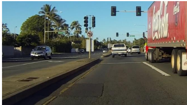
Figure 8-59. Untreated edges in a semi-permanent patch.
