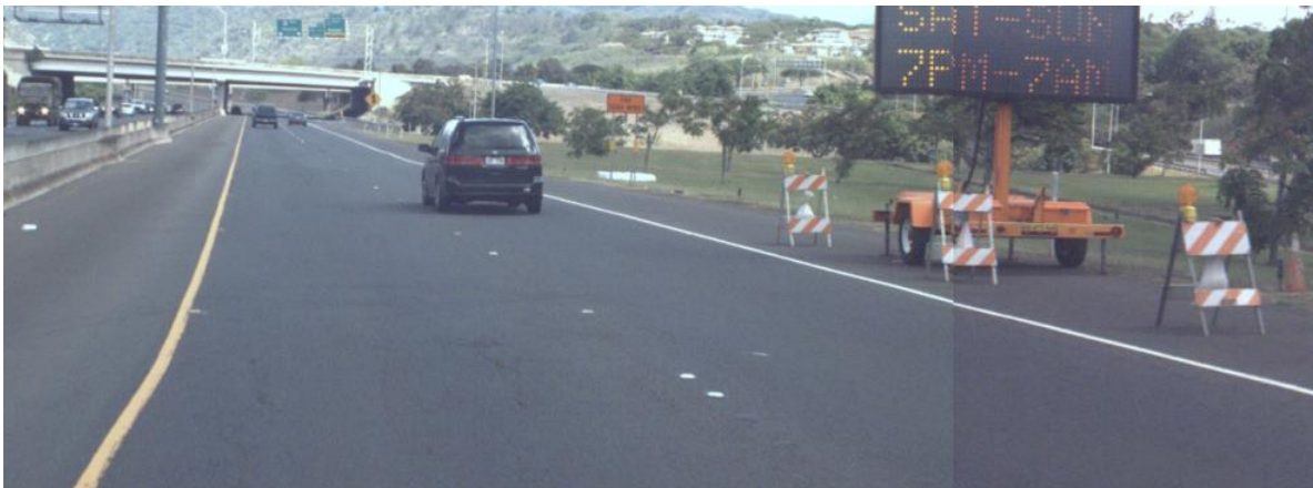
Figure 7-2. Example of higher deterioration on the inside lane (Route H-3, MP 0.108).
