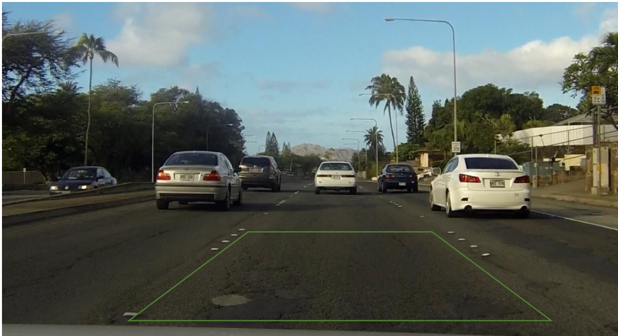
Figure 4-45. Challenges when attempting to quantify areas with raveling.
