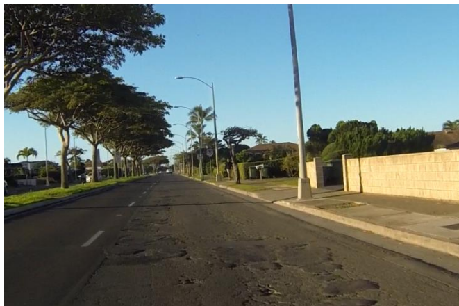
Figure 8-61. Ineffective throw and roll patching.
