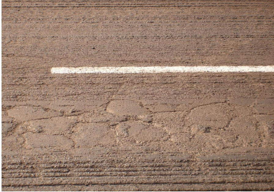
Figure 4-25. Existing cracking over which the overlay was applied on a section of route 7101.
