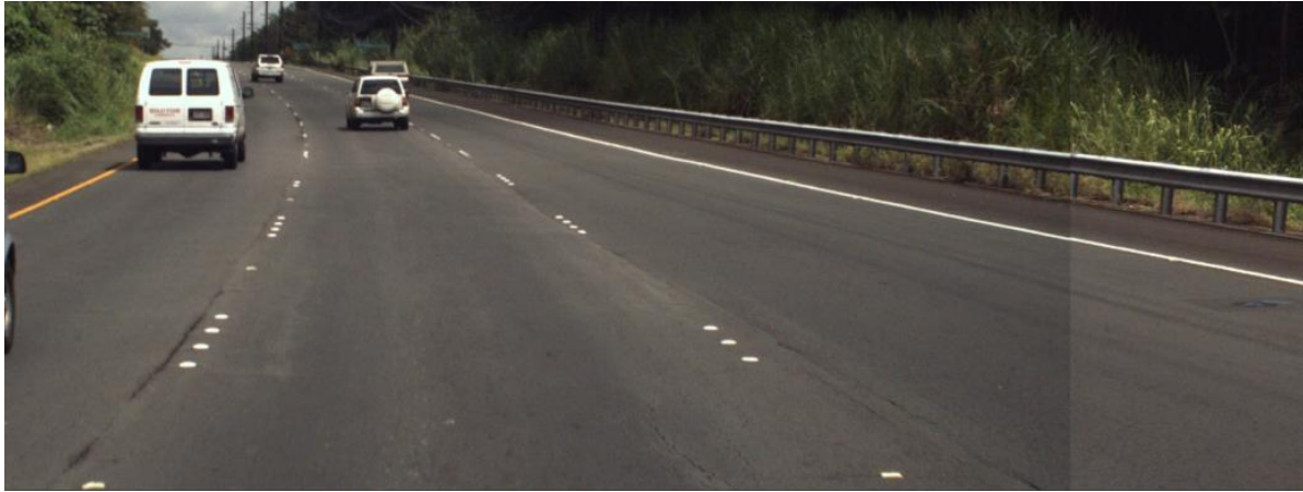
Figure 7-3. Example of center lane with more deterioration than the rightmost lane (Route 11, MP 6.478).
