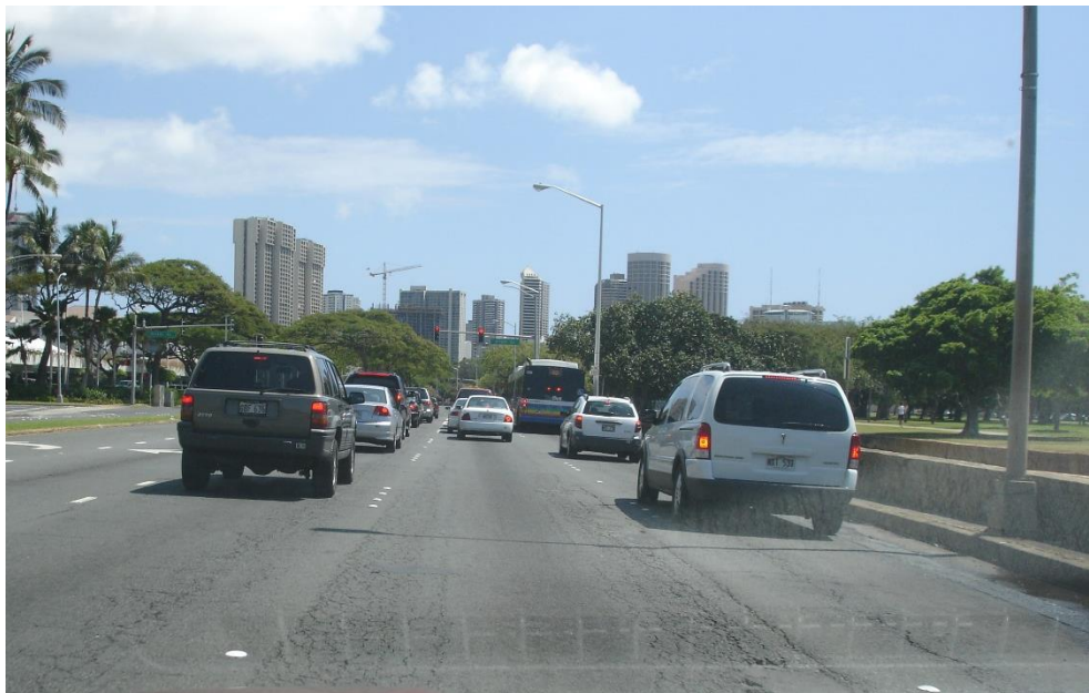
Figure 5-16. Example of section exhibiting fatigue cracking.
