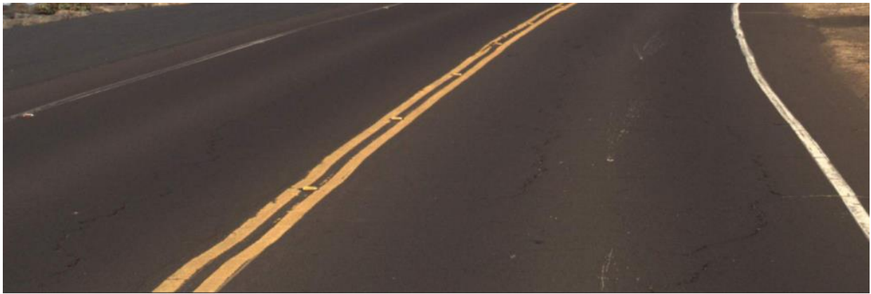
Figure 7-6. Fatigue cracking on Route 50, MP 25.208 in 2012.
