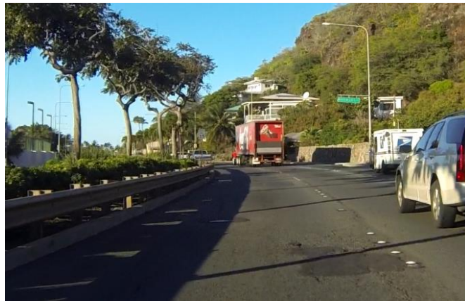
Figure 8-60. Questionable smoothness of throw-and-roll patches in larger potholes.
