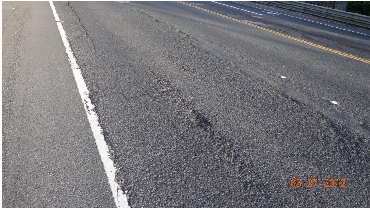
Figure 4-42. Substantial loss of aggregate (Kalaniana'ole Highway).
