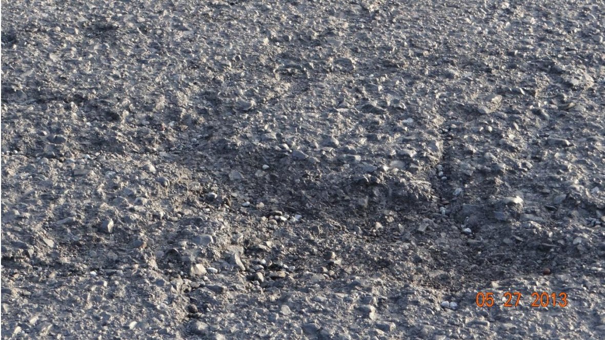
Figure 4-43. Close up illustrating the disintegration of the pavement surface and the loose aggregate.
