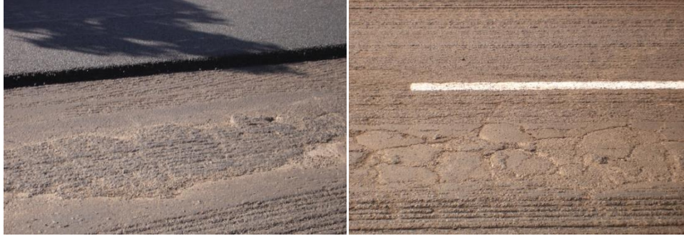
Figure 8-75. Unsuitable conditions for thin hot-mix overlays.
