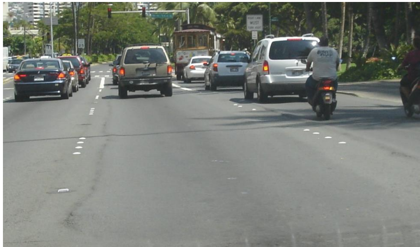
Figure 5-19. Section with center and right lanes exhibiting noticeable rutting in the mix.
