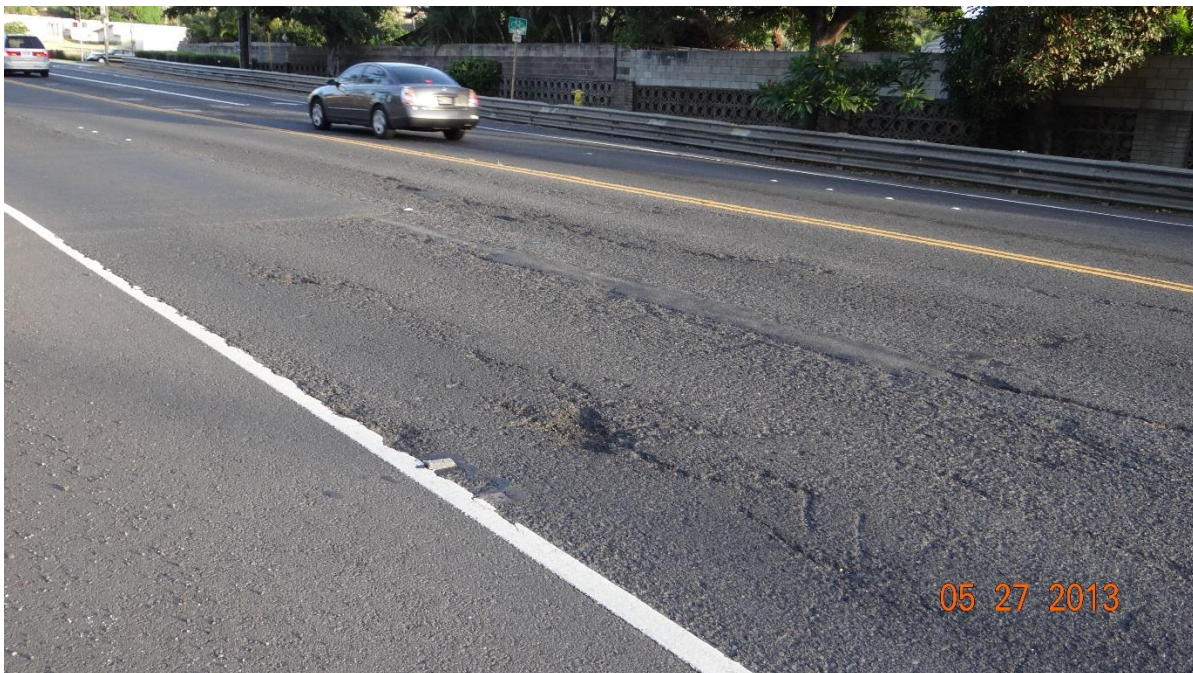
Figure 4-44. Another example of severe raveling on Kalanianaʻole Highway.
