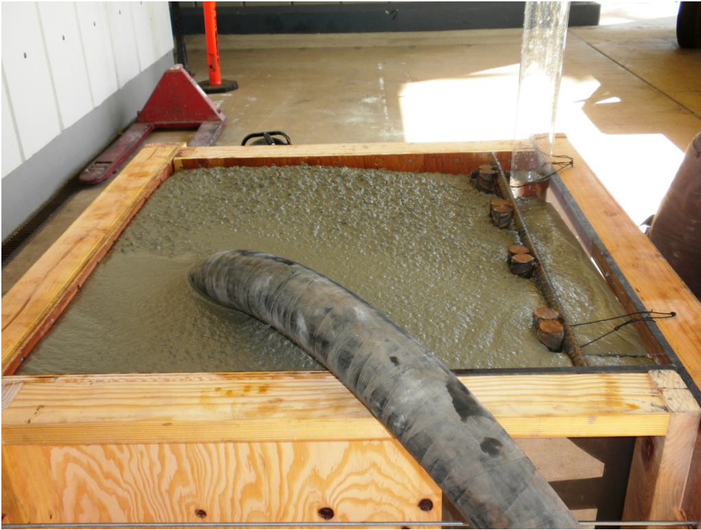
Figure 3: Placement of SCC by pump hose at bottom of form behind reinforcing cage
