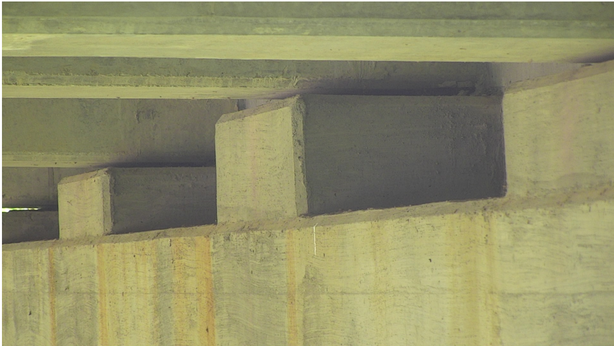
Figure 5.21: Bearing unable to see sufficiently #2.
