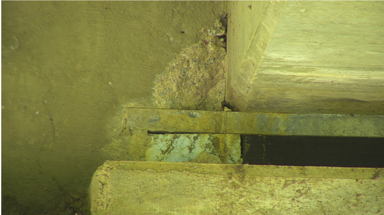
Figure 5.20: Bearing unable to see sufficiently #1.
