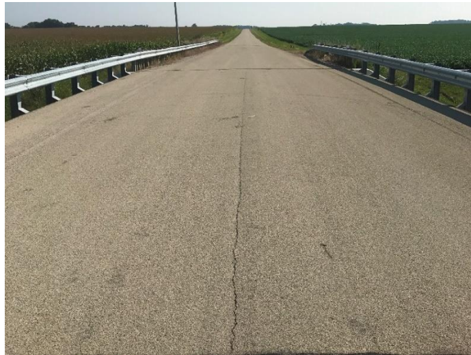
Figure 3: Sollars Road Bridge Asphalt Crack
