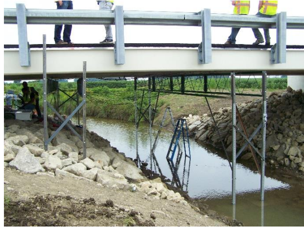
Figure B12: Instrumentation Frames
