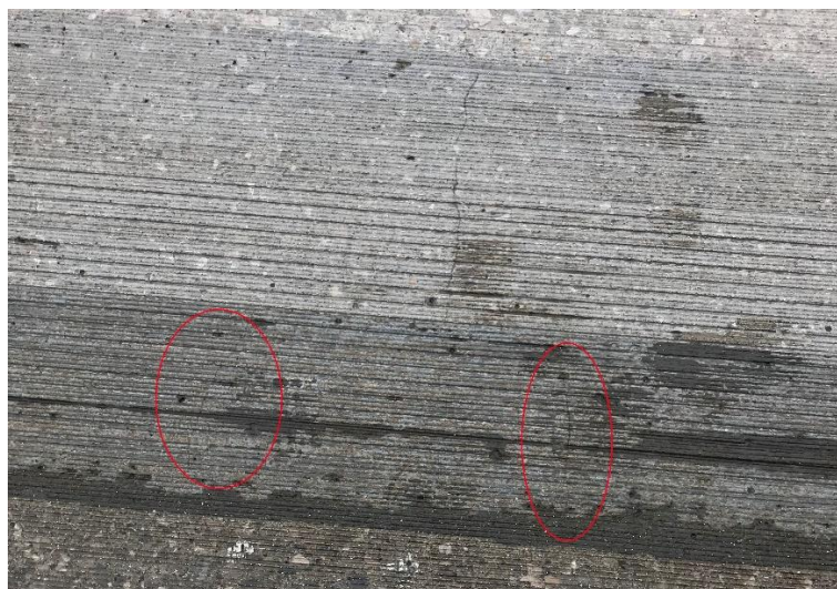
Figure C15: Cracks in UHPC and Deck
