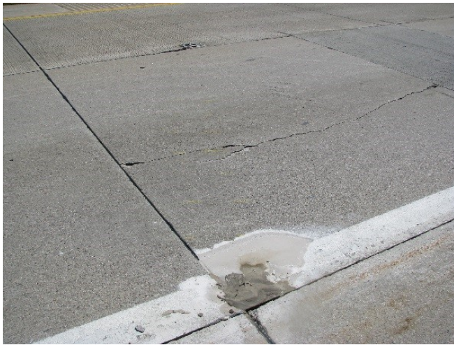
Figure 13: Midslab longitudinal cracking in surveyed Michigan sections
