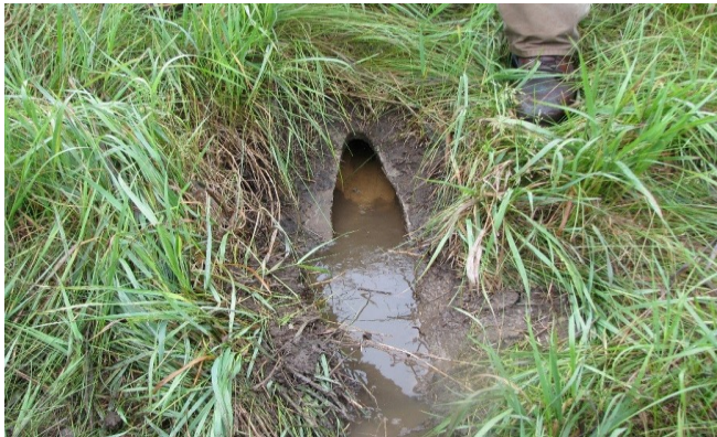
Figure 11: Plugged edge drain near surveyed Michigan sections
