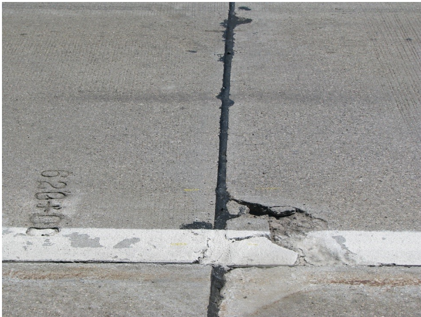
Figure 14: Wider working joint exhibiting distress in surveyed Michigan sections
