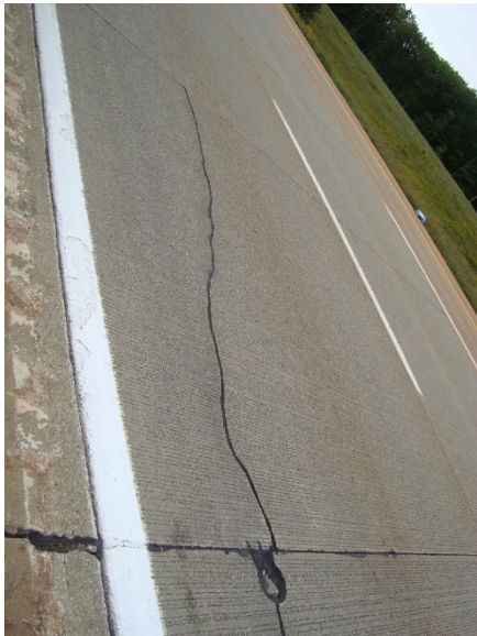
Figure 110: Random longitudinal crack on I-75 near West Branch, Michigan.
