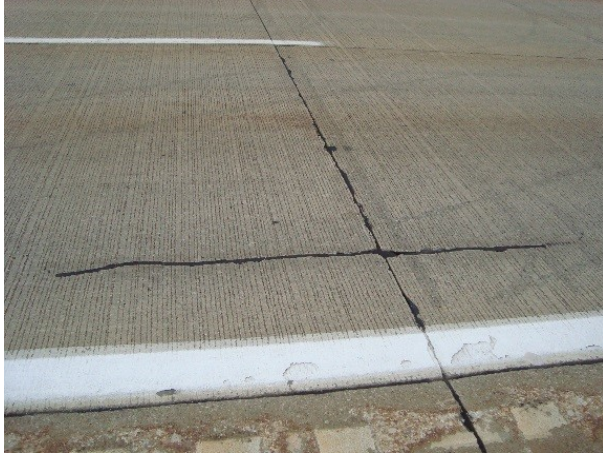
Figure 12: Longitudinal (or diagonal) cracking in the wheel path in sections surveyed in Michigan
