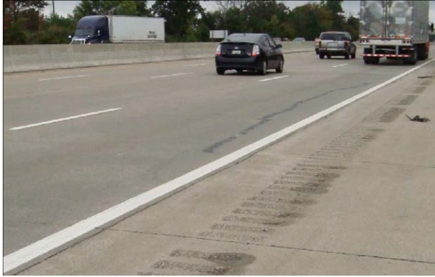
Figure 10: Longitudinal cracking due to erosion of the HMA interlayer in surveyed Michigan sections
